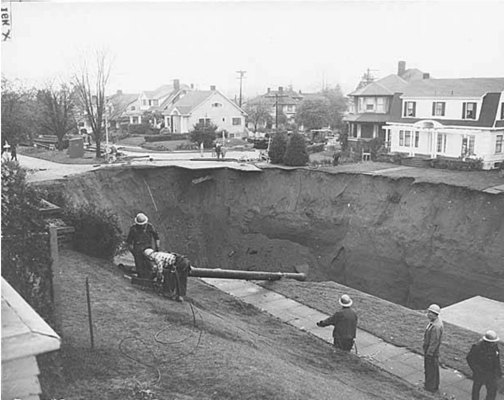
Ravenna Avenue sewer cave-in at 16 th & Ravenna Blvd, 1957 (Seattle Municipal Archives)
