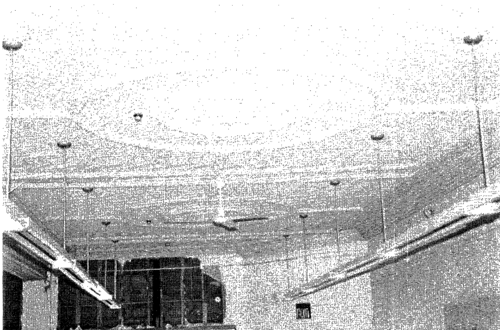
Figure 6: Plaster ceiling modillions, south half of original (corner) bank storefront, view east towards angled entryway.
