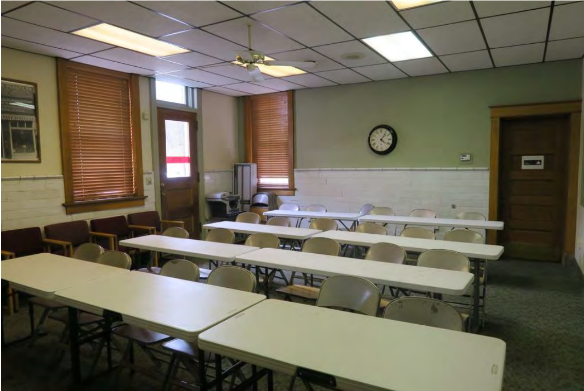
16 of 35: Interior-south end of original general waiting room, current classroom, camera looking south east.
