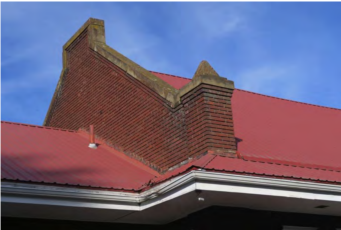
11 of 35: Parapet at south end of main lobby center section; camera looking west.
