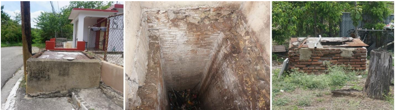
On the left, service manhole to the supply channel, located on a sidewalk of the El Ojo Community. In the center, detail of the service shaft inside a manhole. Right, manhole which features an advanced degree of damage by erosion, located in the backyard of a house.
