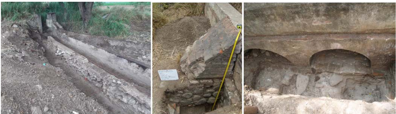
Left; view of the Hacienda Florida channel at its origin as it left the distribution module, facing northeast. Center; Detail of an abutment. Right; segment of the channel on arches. Note the stone pavement under the channel.
