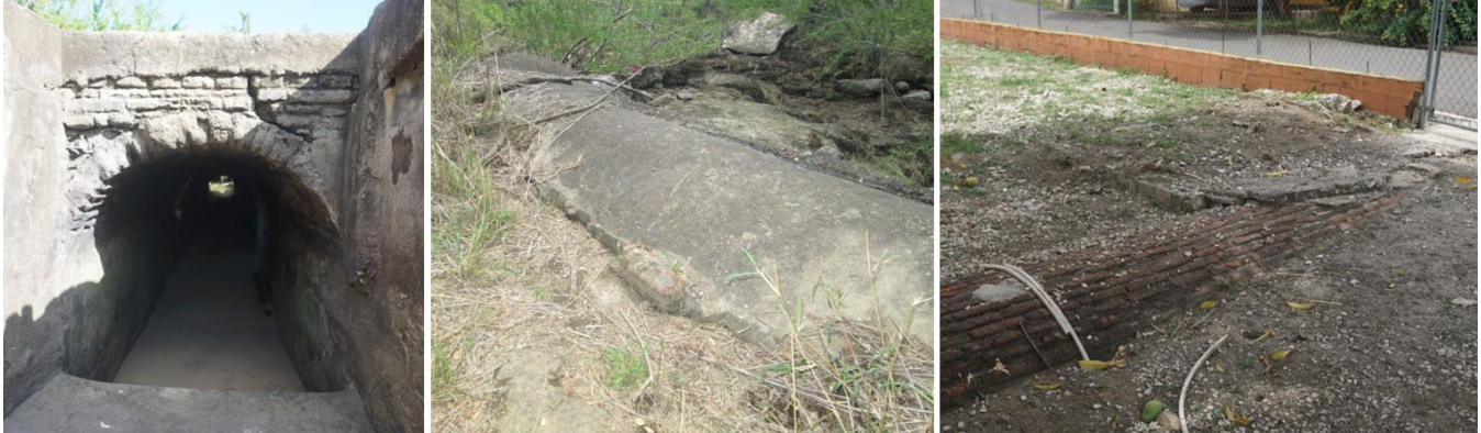
On the left, entrance to the Supply channel at the low-waters module, looking south from within the inlet. In the center, vaulted segment of the supply channel that runs along the surface in the area of the dam. Notice the concrete plastering over the vault. On the right, view of the channel as it emerges to the surface, in the backyard of a property of the El Ojo Community. Note that the vault does not have plastering.
