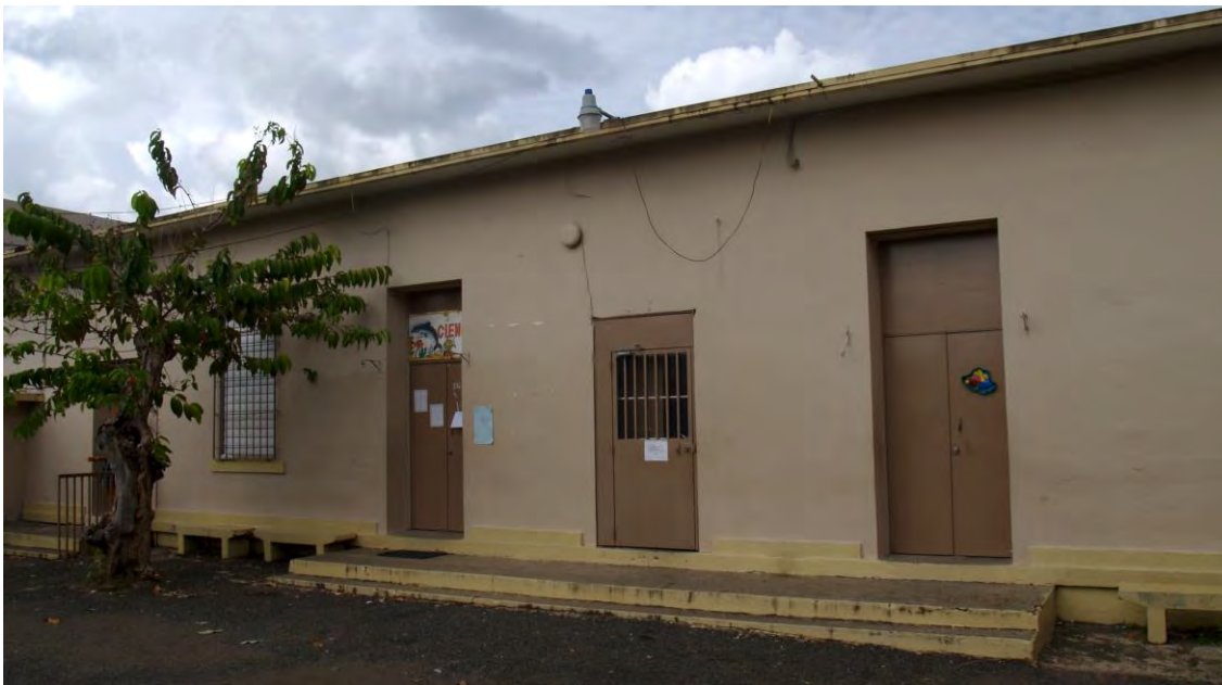
Figure 4. Eugenio M. de Hostos’ rear (southern) façade. The metal door with the bars was the rear entrance to the central hallway. The metal doors on both sides were originally windows, expanded as doorways to serve the two classrooms to which they belong. (Source: Juan Llanes Santos, 2014)
