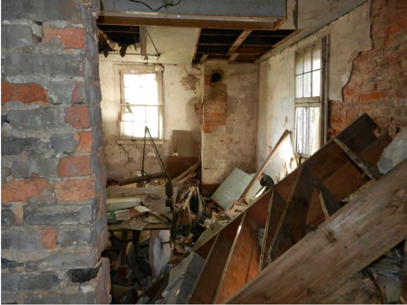
Photo 17: WV_JeffersonCounty_Feagans' Mill_017 Feagans' Mill, First Floor, West Wall Looking into Creamery (North and West Walls)
