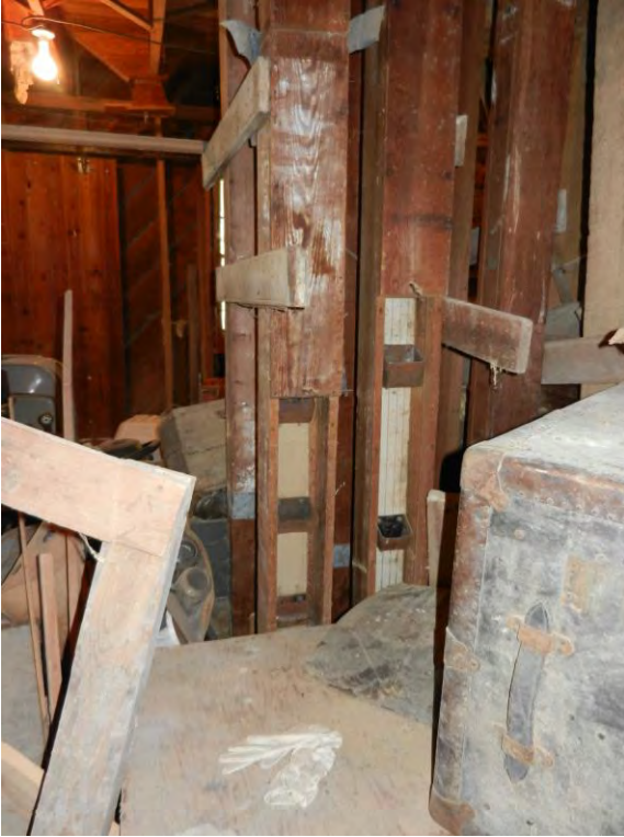
Photo 29: WV_JeffersonCounty_Feagans'Mill_029 Exposed view of elevator cups to raise grain from basement to upper floors
