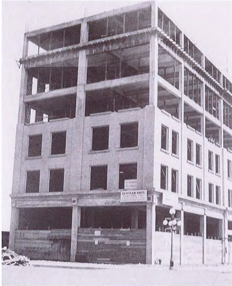
Figure 3: Construction Photo, 1914, when the 3 rd through 6 th stories were in process. Note the central beam and joists that comprise the module of the concrete frame. The small sign in the first story window reads "Frederick Hurst, Architect".
