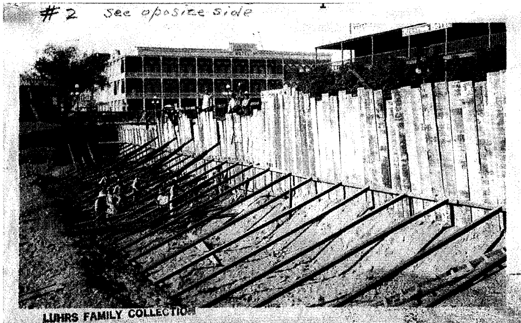
Figure 8: Wood formwork for the Luhrs Central Building. To the right in the photo is the Kersting Hotel. The three-story building in the rear of the photo is the Commercial Hotel. The lot between the two buildings would become the site of the Jefferson Hotel. Photo Fall 1913. (ASU Hayden Library, Luhrs Reading Room, CP LFPC 533)
