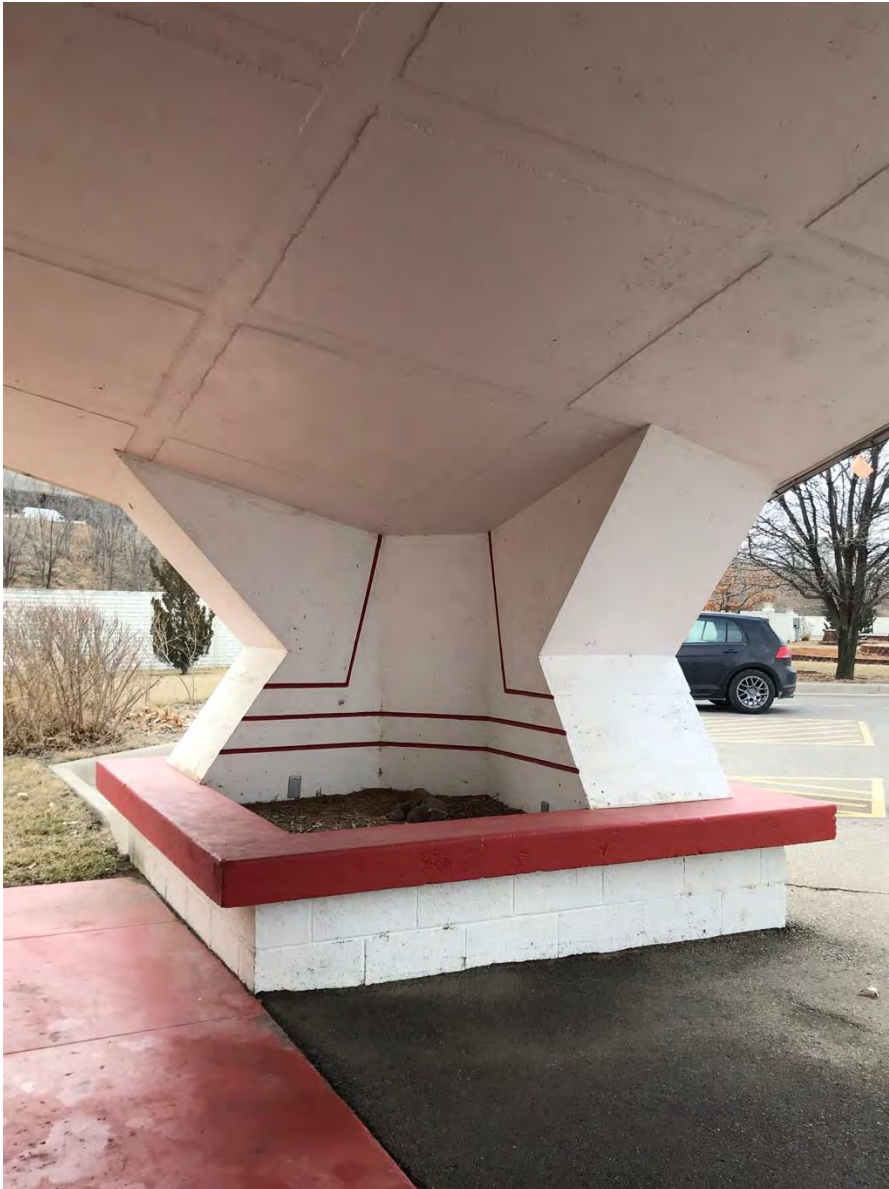
Photo: One of the two large column planters at which the roof shell terminates.
