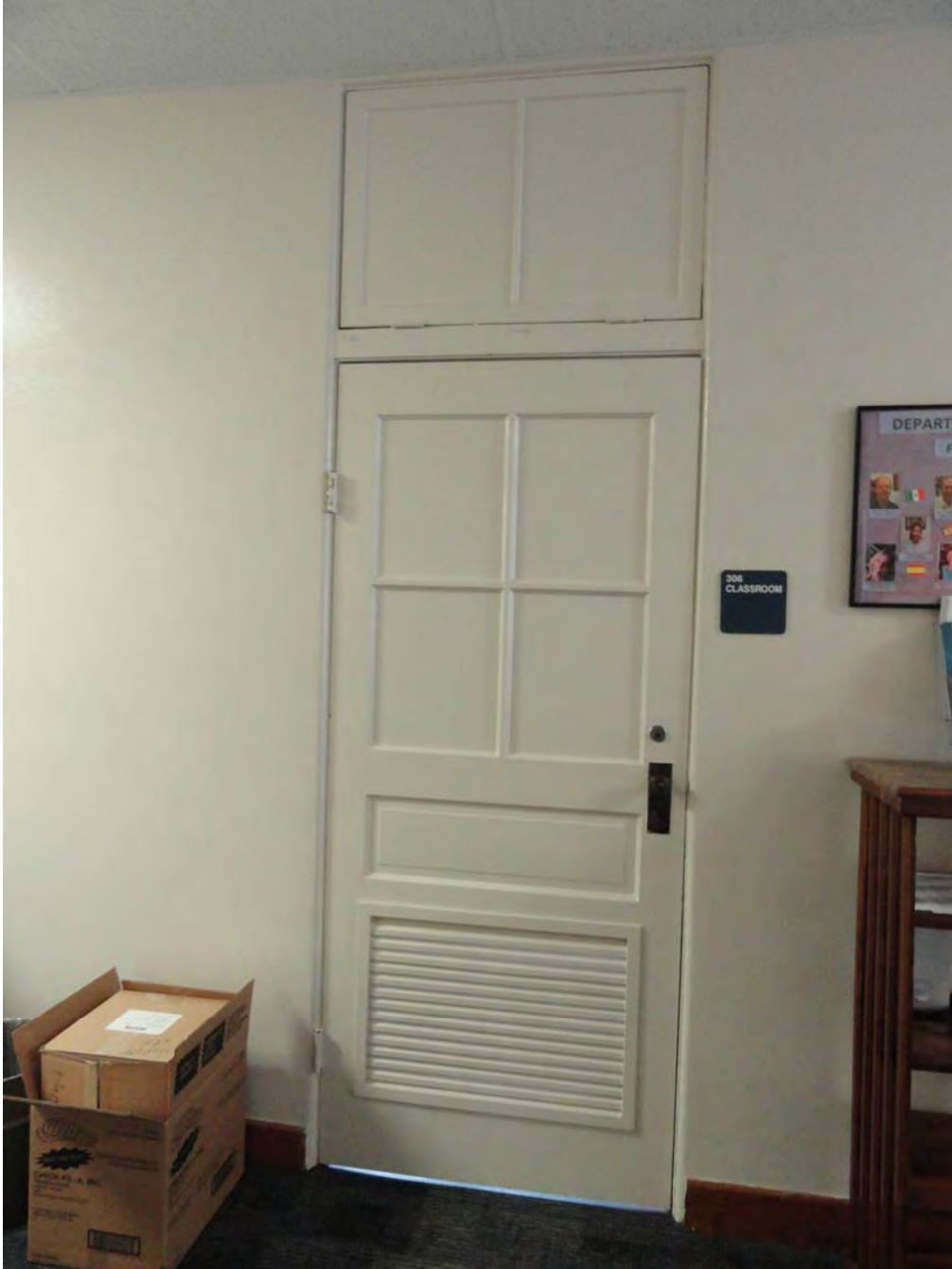
Photo 17: door to hallway with original transom and louvered ventilation panel Photographed by Maria Pfeiffer, May 2015
