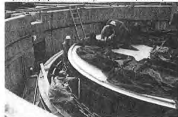
CRUSHING STICKS of 3/4-inch plywood, held in the 1/2-inch air gap between the stator and rotor pole faces, assured proper centering of the rotor as it was lowered. (FIGURE 8)
