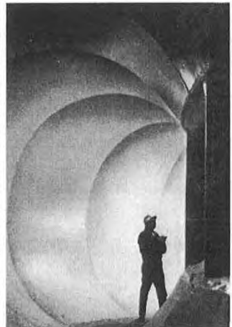
FROM THE 18-FOOT diameter penstock, water will fill the scroll case, surround the stay ring and wicket gates. (FIGURE 5)
