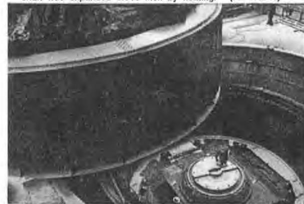
READY FOR INSTALLATION, the 330-inch diameter rotor will be lowered into the 331-inch diameter stator, the expanded keyway mated to the key. (FIGURE 7)
