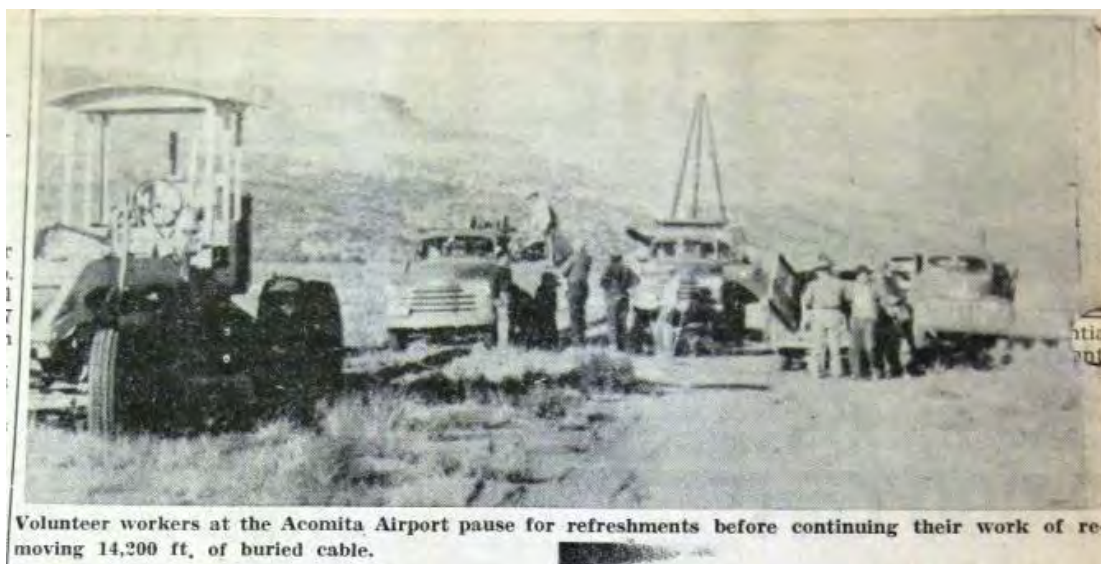
Figure 7. "Volunteer workers at the Acomita Airport pause for refreshments before continuing their work of removing 14,200 feet of cable."
