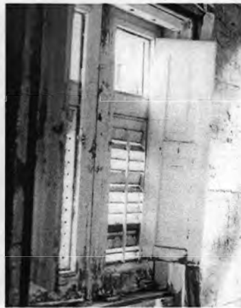
Fig. 10 Photos original wooden windows 10
