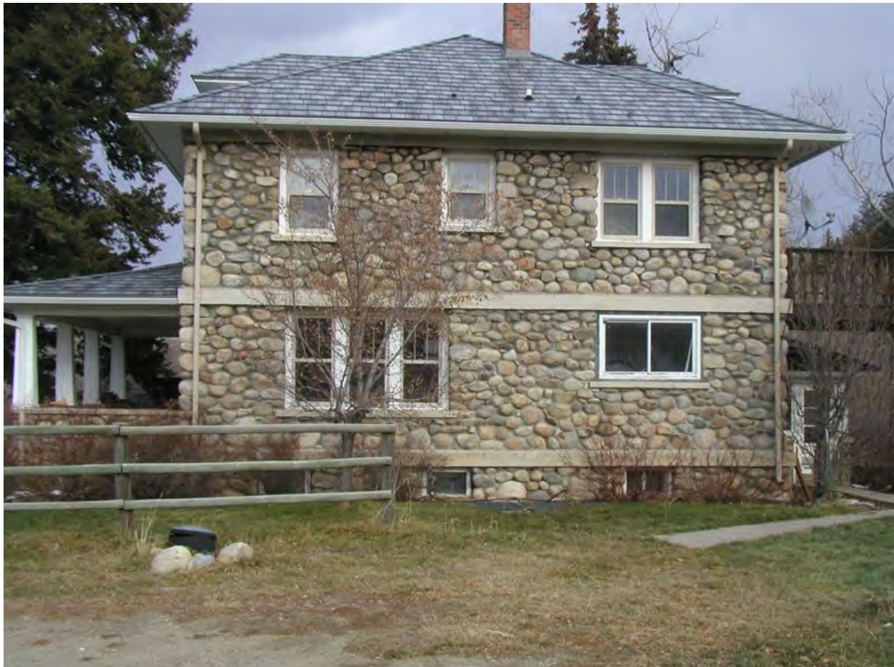
Description and view of camera: South elevation, view to north Photograph: MT_StillwaterCounty_CharlesGladysPeltonHouse_0008
