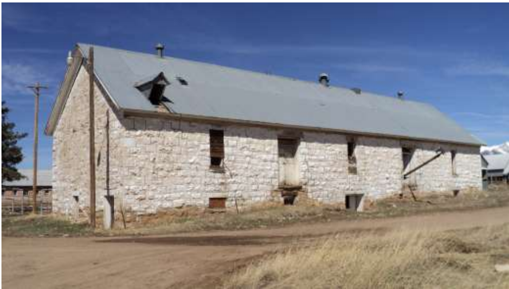
Figure 8-6. Quartermaster's Storehouse, Old Fort Lewis, Colorado Southeast Side Photographed by Lillian Makeda, March 16, 2011
