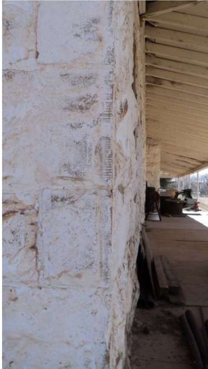
Figure 8-8 Guardhouse, Old Fort Lewis, Colorado Masonry Detail, Southwest Corner Photographed by Lillian Makeda, March 16, 2011
