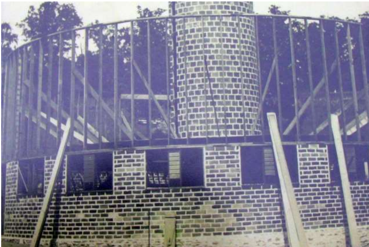
Photograph of the Albert and Minna Ten Eyck Round Barn under construction from the southwest; circa 1922. Image courtesy of Robert Ten Eyck.
