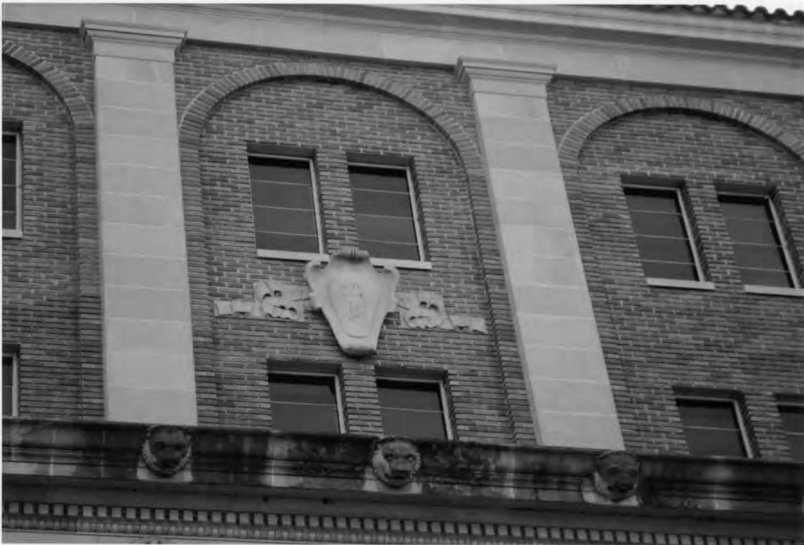
10. John C. Calhoun State Office Building 1015 Sumter Street, Columbia Richland County, South Carolina
