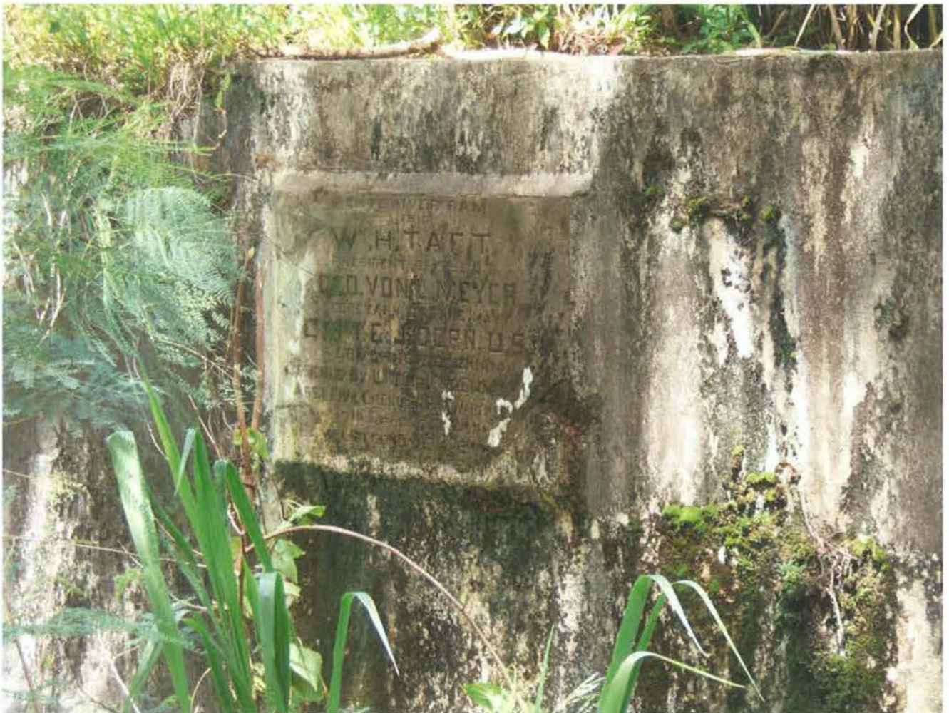
Figure 2: Concrete Dedication Plaque on the western wall of the Fonte River Dam facing south. The plaque reads: FONTE RIVER DAM / 1910. / WM. H. TAFT. / PRESIDENT OF THE US / GEO. VON L. MEYER / SECRETARY OF THE NAVY / CAPT. E. T. DORN, U.S.N. / GOVERNOR OF GUAM / DESIGNED BY L. M. COX CIVIL ENGINEER U. S. (Broken off after S) / ASST. CIVIL ENGINEER R. M. WARFIELD (Broken off...previously noted U.S. before first break) / IN CHARGE OF WORK / COMPLETED BY C. A. BOSTROM / ASST. CIVIL ENGINEER
