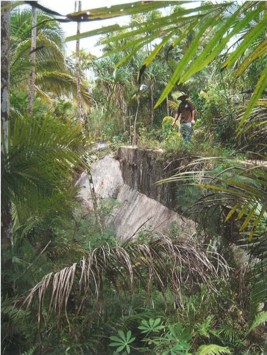
Figure 3: A view of the western wall of the Fonte River Dam looking south east.
