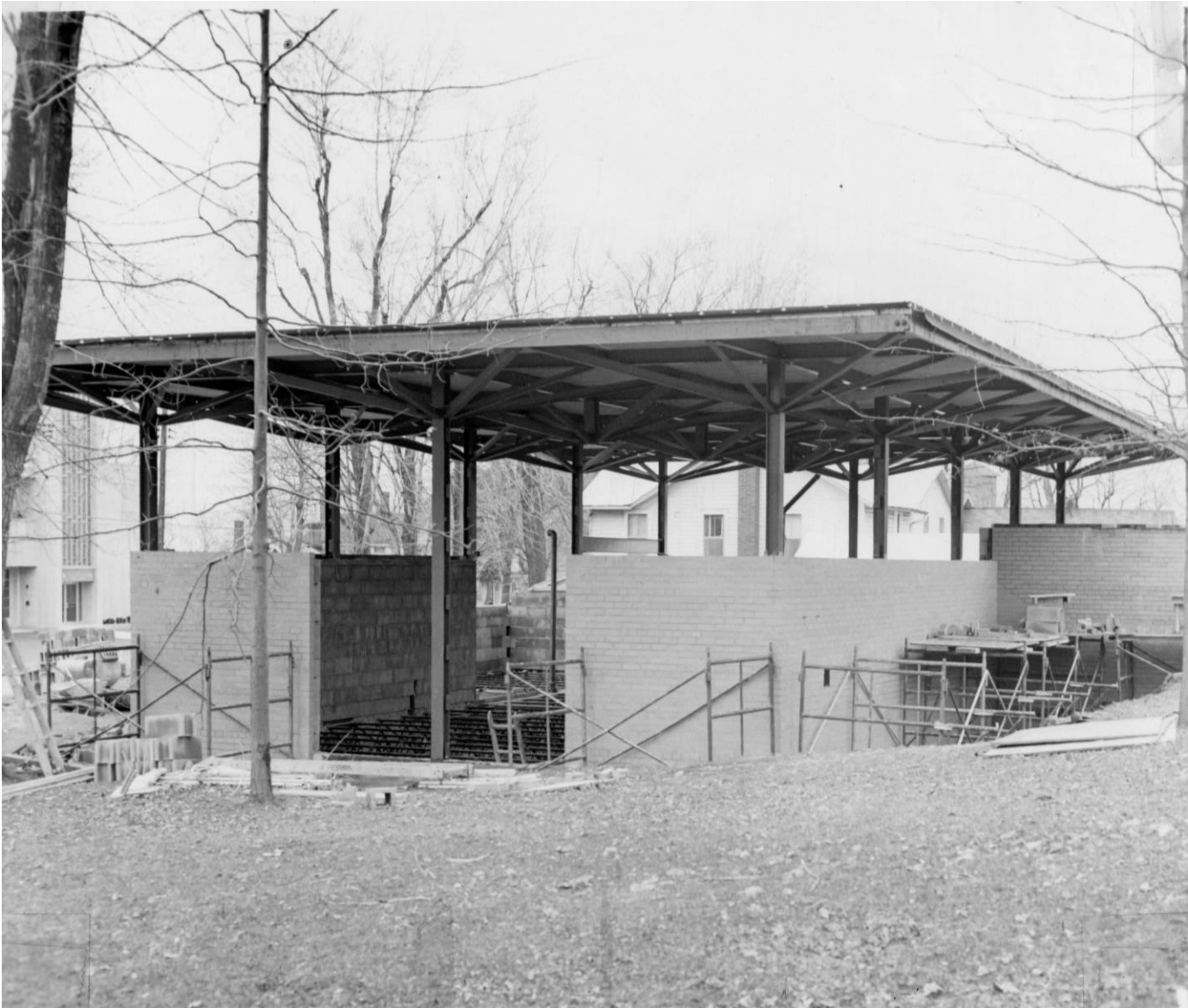
Construction photograph showing open plan of the library and roof support system. From the collection of the Edith B. Ford Memorial Library Archive.
