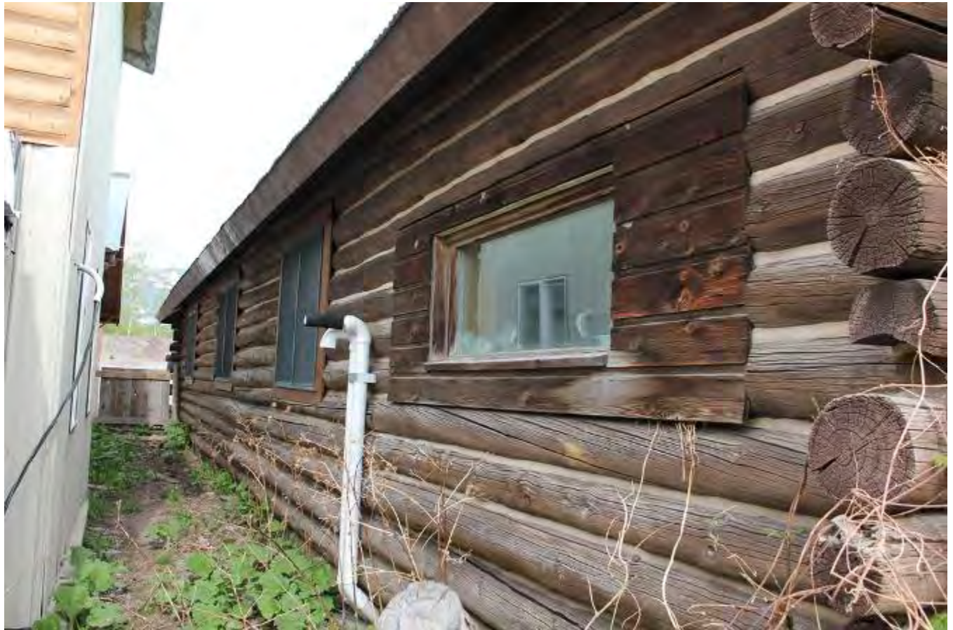
Description of Photograph(s) and number: South (side) elevation. View from southeast corner. MT_GlacierCounty_GlacierParkWomen'sClub_0007 of 0011.
