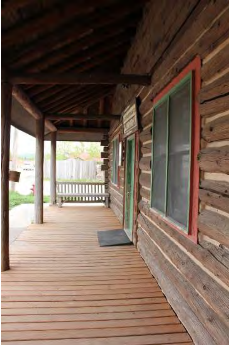
Description of Photograph(s) and number: Detail of west (front) elevation porch. MT_GlacierCounty_GlacierParkWomen'sClub_0005 of 0011.
