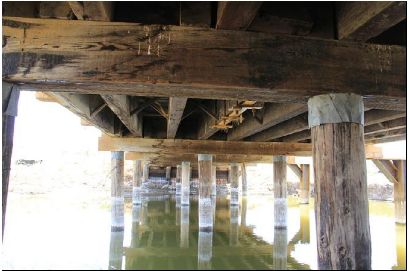
Photo 0007. Cottonwood Creek Bridge. Detail of underside of deck. View to the south.
