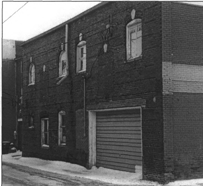
Darker rowlock brickwork pattern, rear wall, 424 West Main (Photo by Jim Jacobsen, January 14, 2005)
