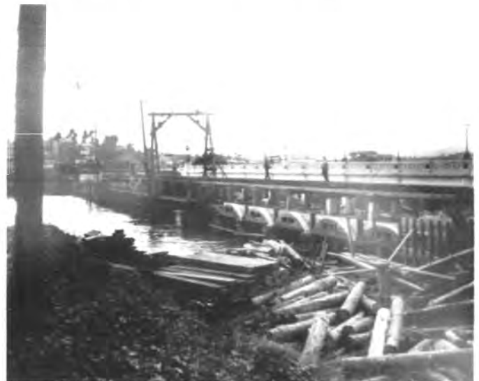
Figure 8. Placement of precast concrete arcade in the north section as seen from the San Juan Islet. January 16, 1932.
