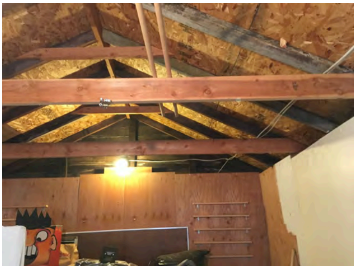
Figure 15: New OSB on roof, rafter ties, collar ties and new 2x ridge board
