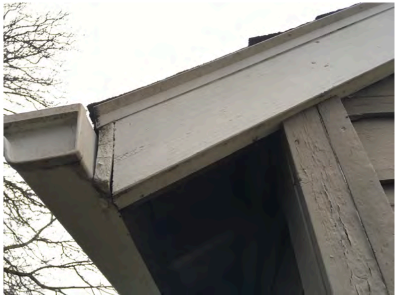
Figure 14: (All) Defects in materials and workmanship on siding and trim, note also the different corner board conditions
