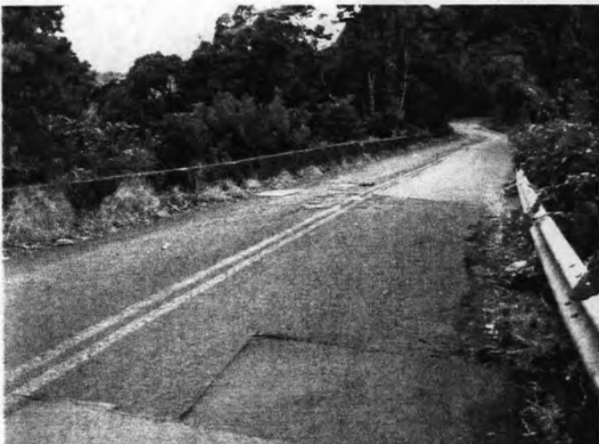
Figures 17 and 18: “Hogsback”, near Mile Marker 4.0 Basalt (lava rock) retaining wall at Hogsback.
