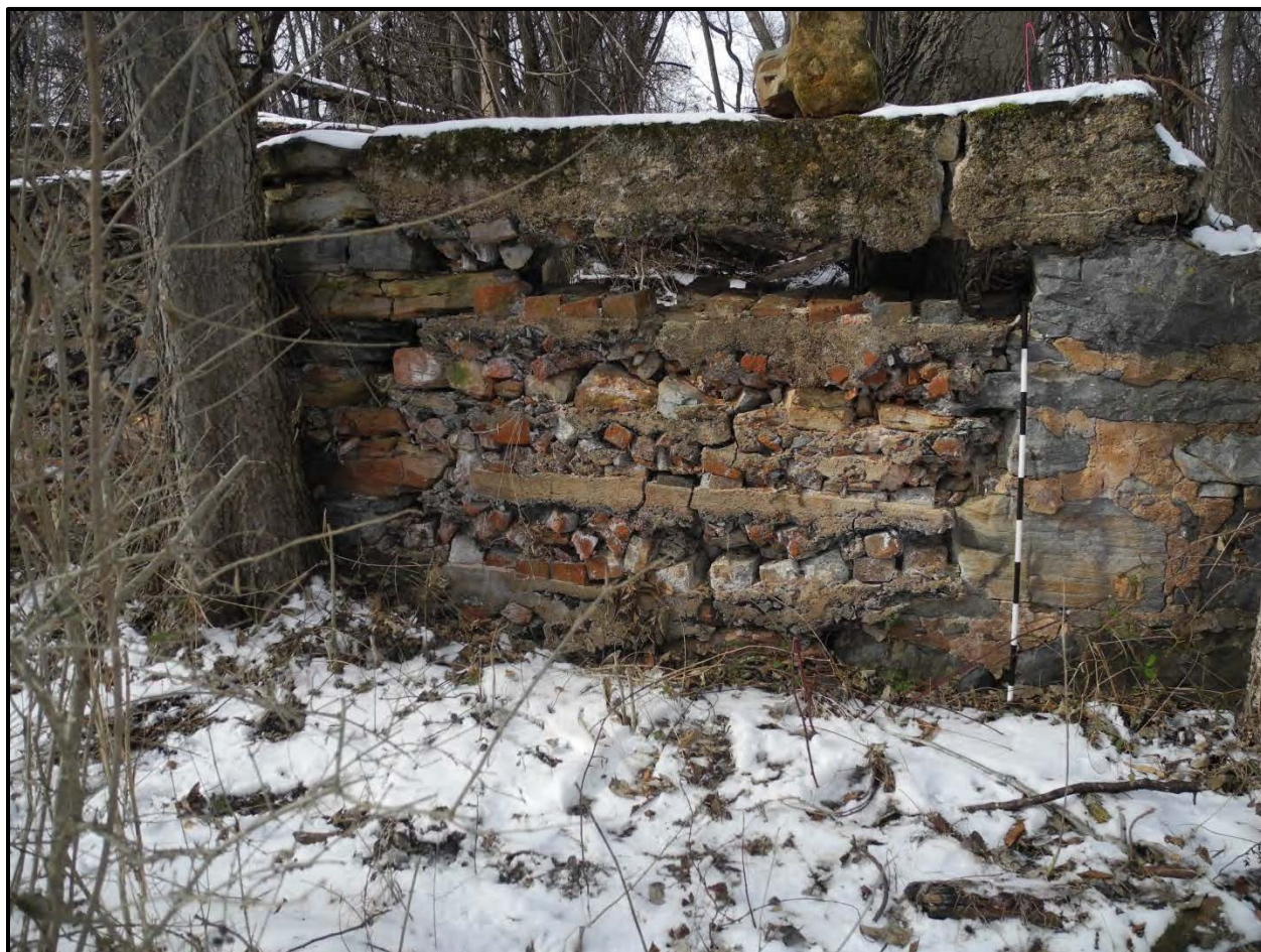
Figure 18. Barn Site, Brick and mortar-filled opening in front (east) wall (scale = 1 meter).
