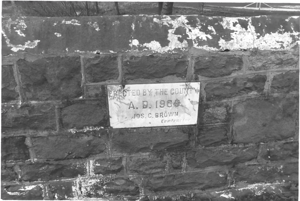
Bridge Date Stone, Dr. Smith's Sanitarium Site, Egg Harbor City, Atlantic County, NJ (# 4 of 14)
