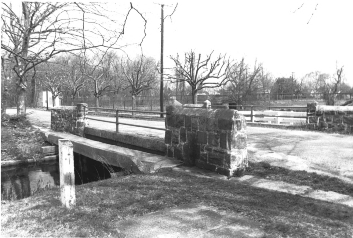
Bridge . Dr. Smith's Sanitarium Site, Egg Harbor City, Atlantic County, NJ (#5 of 14)
