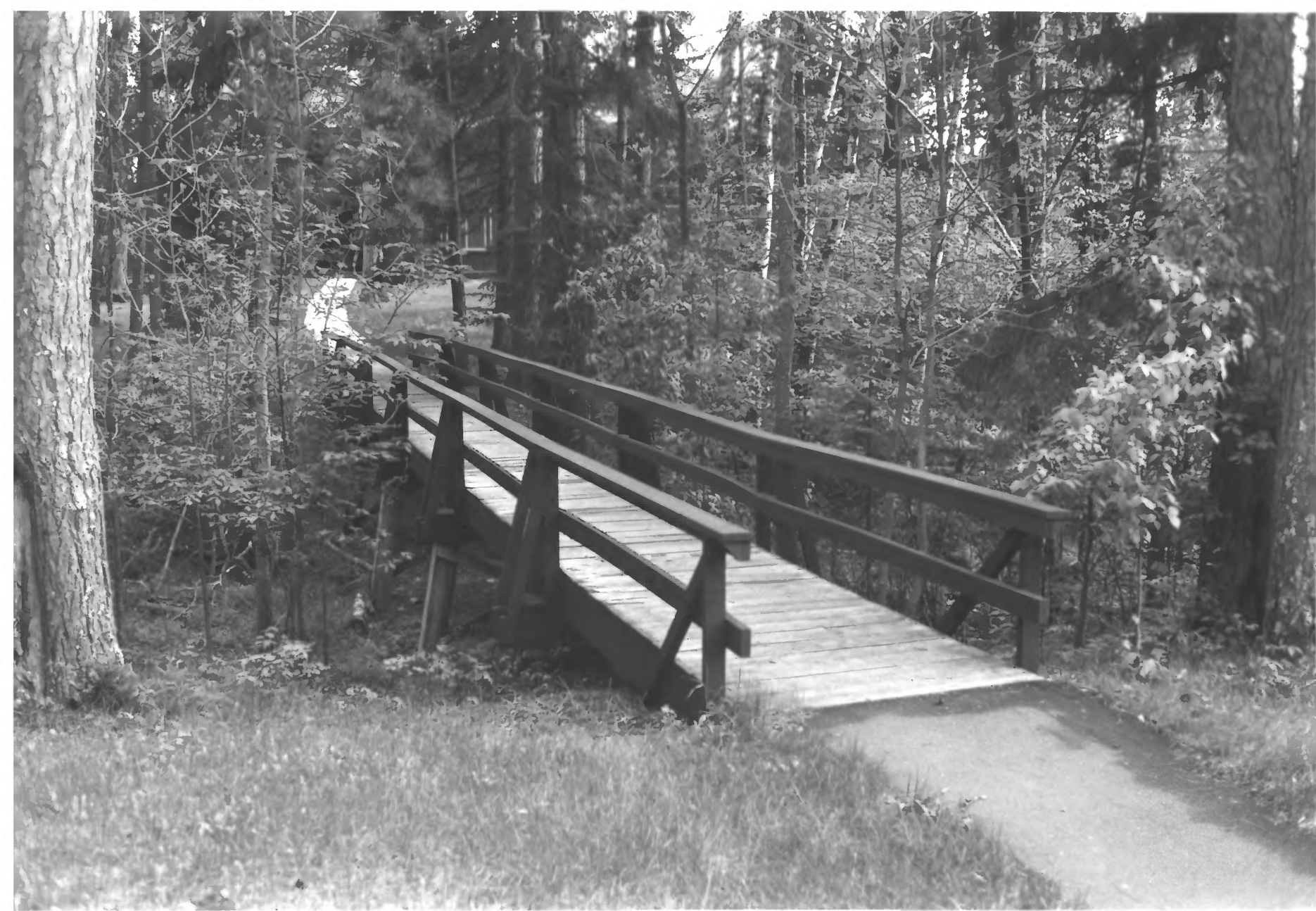
ITASCA STATE PARK CCC/WPA/RUSTIC STYLE HISTORIC RESOURCES CLEARWATER & HUBBARD COS., MN STRUCTURE #12 PHOTO I.D. 09773#2 (NON-CONTRIBUTING)
