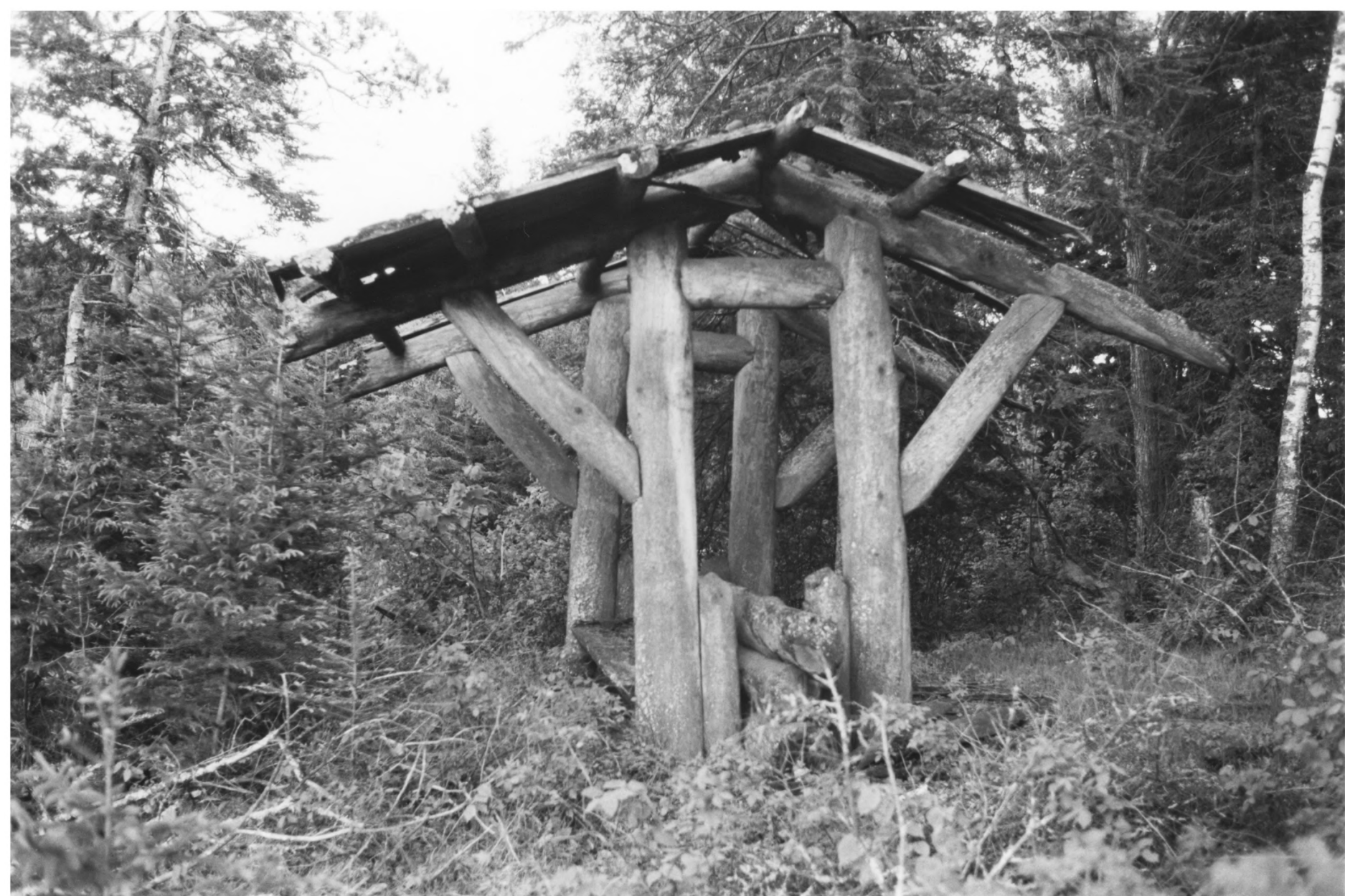
ITASCA STATE PARK CCC/WPA/RUSTIC STYLE HISTORIC RESOURCES CLEARWATER & HUBBARD COS, MIN. STRUCTURE # 31 PHOTO I. D. 09785 # 12A
