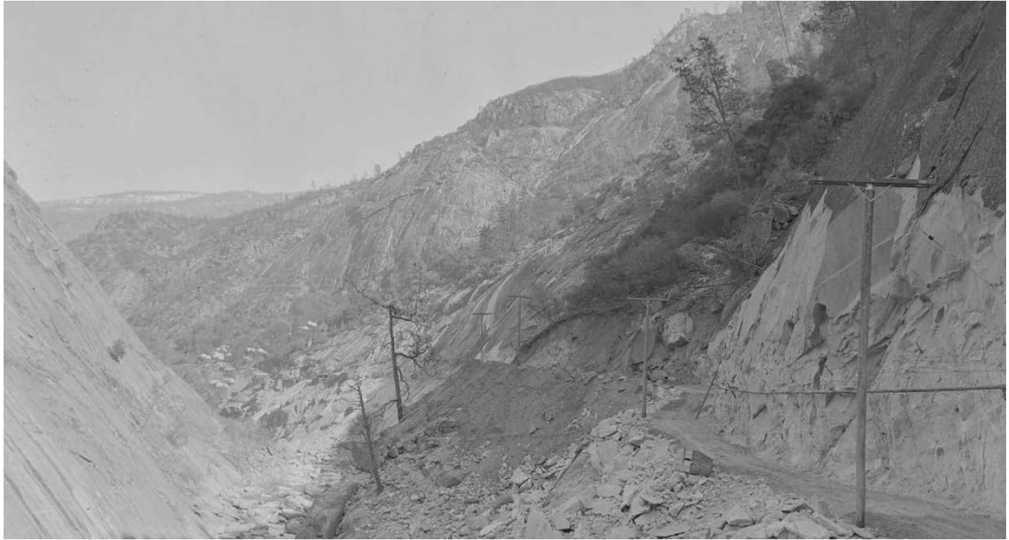
Figure 126: Million Dollar Mile Road partially completed, 1922. Image No. SCE-02-07574, Huntington Digital Library.
