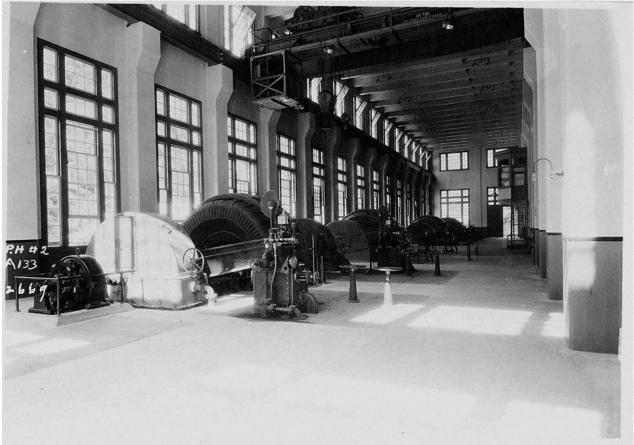
Figure 25: Interior of generator floor for Powerhouse No. 2, 1925. Image No. SCE-02-12669, Huntington Digital Library.
