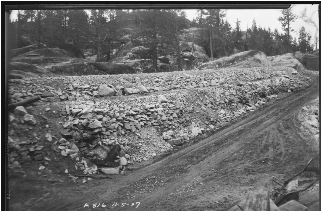
Figure 133: Mono-Bear Road alignment paralleling siphon at left, 1927. Image No. SCE-02-14752, Huntington Digital Library.
