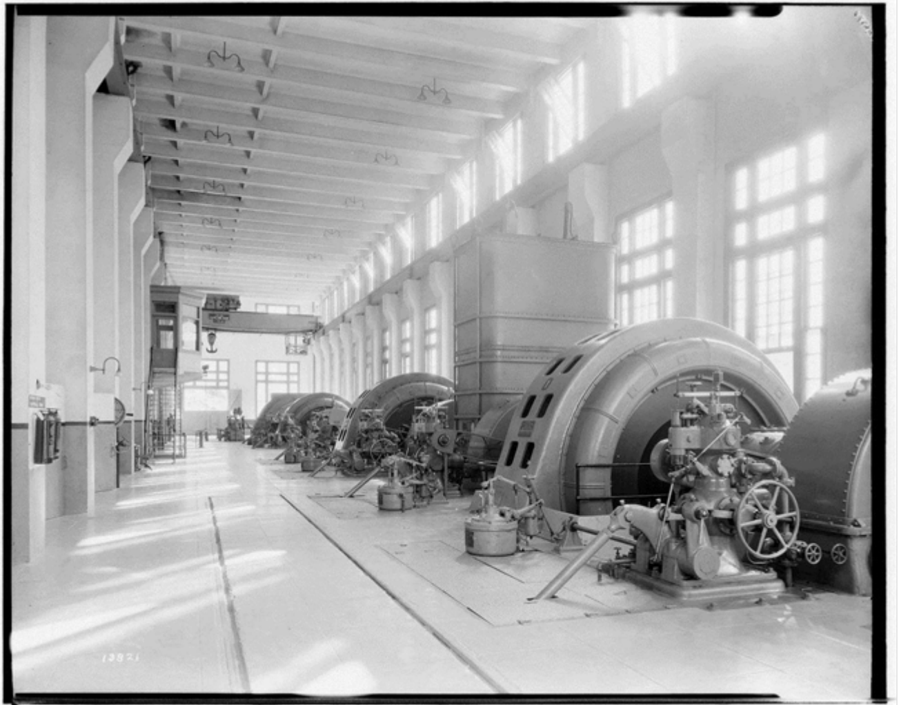
Figure 14: Interior of Powerhouse No.1 generator floor with 4 units installed, 1926. Image No. SCE-02-13821, Huntington Digital Library.
