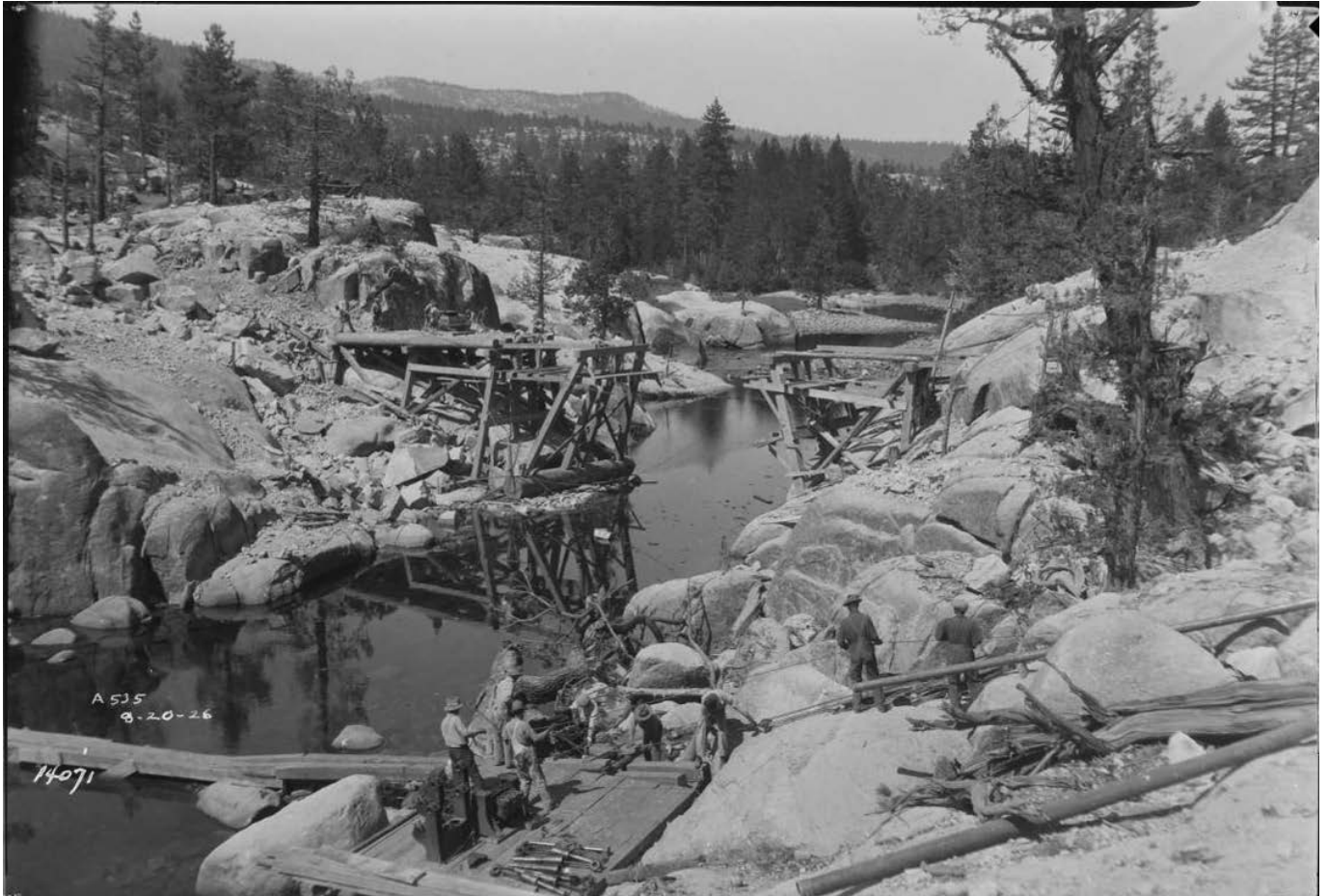
Figure 132: Mono-Bear Road San Joaquin River Bridge construction, 1926. Image No. SCE-02-14071, Huntington Digital Library.
