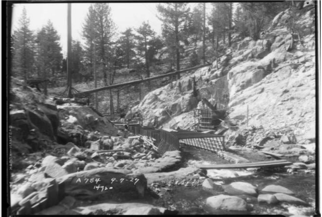
Figure 73: Mono Creek Diversion Dam Construction Site, 1927. Image No. SCE-02-14720, Huntington Digital Library.
