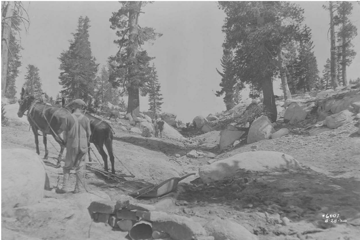
Figure 129: Kaiser Pass Road construction with mules and scrapers, 1920. Image No. SCE-02-06407, Huntington Digital Library.
