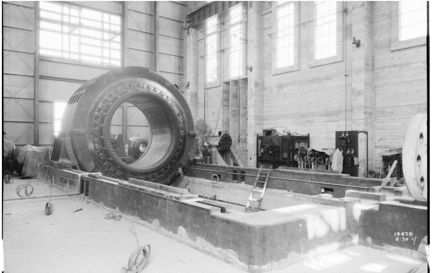
Figure 105: Rector Substation Interior, Frequency Changer being placed, 1927. Image No. SCE-02-14428, Huntington Digital Library.
