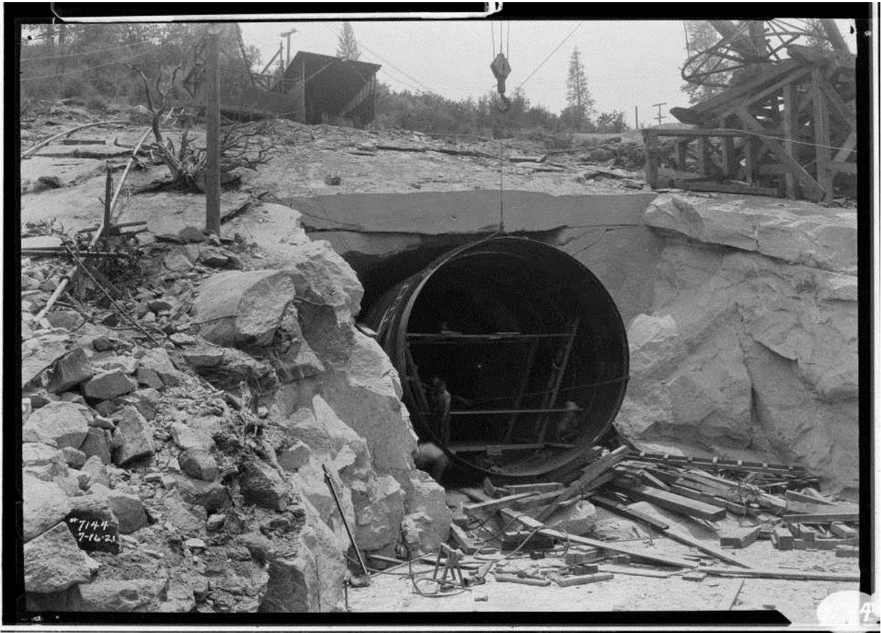
Figure 32: Tunnel No. 8 Outlet, to be connected to surge chamber, 1921. Image No. SCE-02-07144, Huntington Digital Library.
