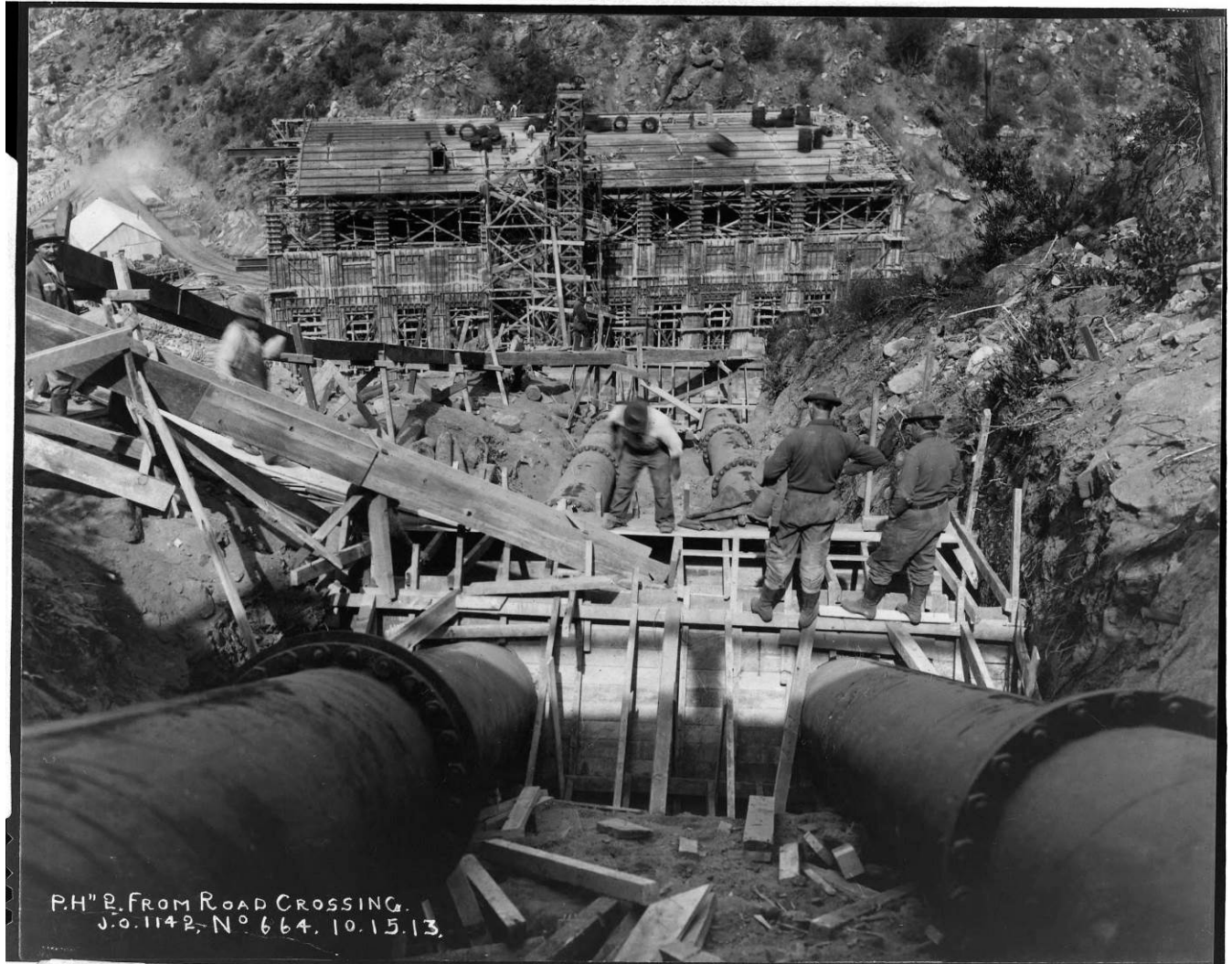
Figure 23: Penstocks for Powerhouse No. 2 looking toward the still-incomplete powerhouse, 1913. Image No. SCE-12-00044, Huntington Digital Library.
