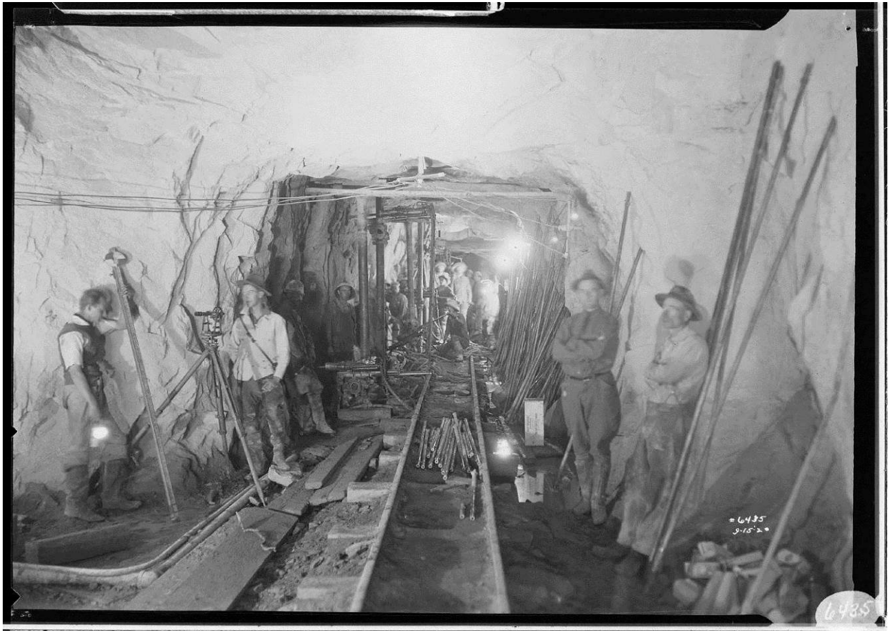
Figure 31: Tunnel No. 8 near Camp 31, depicting crew expanding pioneer bore to full tunnel width, 1920. Image No. SCE-02-06435, Huntington Digital Library.
