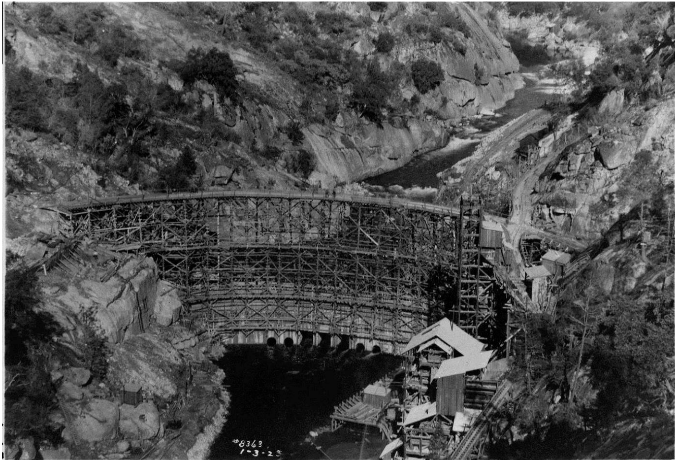
Figure 47: Dam No. 6 under construction looking upstream, 1923. Image No. SCE-02-08363, Huntington Digital Library.
