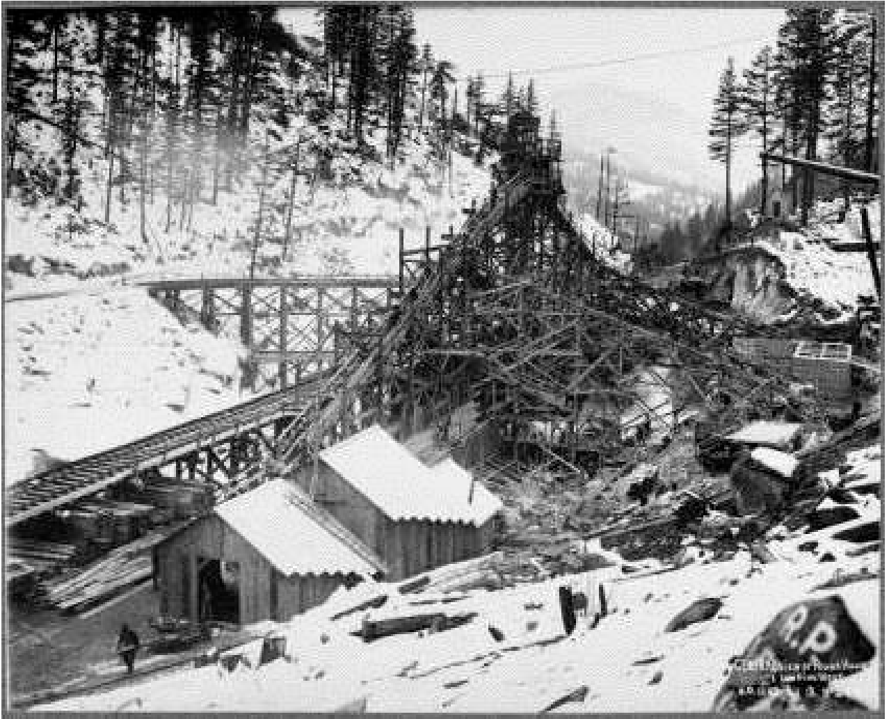
Figure 12: Construction of Powerhouse No. 1 in Big Creek, 1913. Call No. 13 - VOL 002, P071, Huntington Digital Library.
