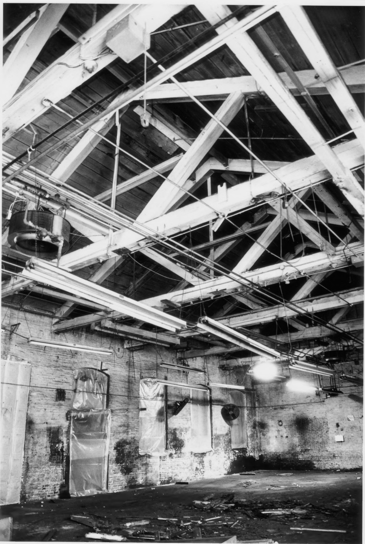
Interior Building 12 looking South Rhode Island TOOL COMPANY Providence, Providence County, Rhode Island Photograph No. 18
