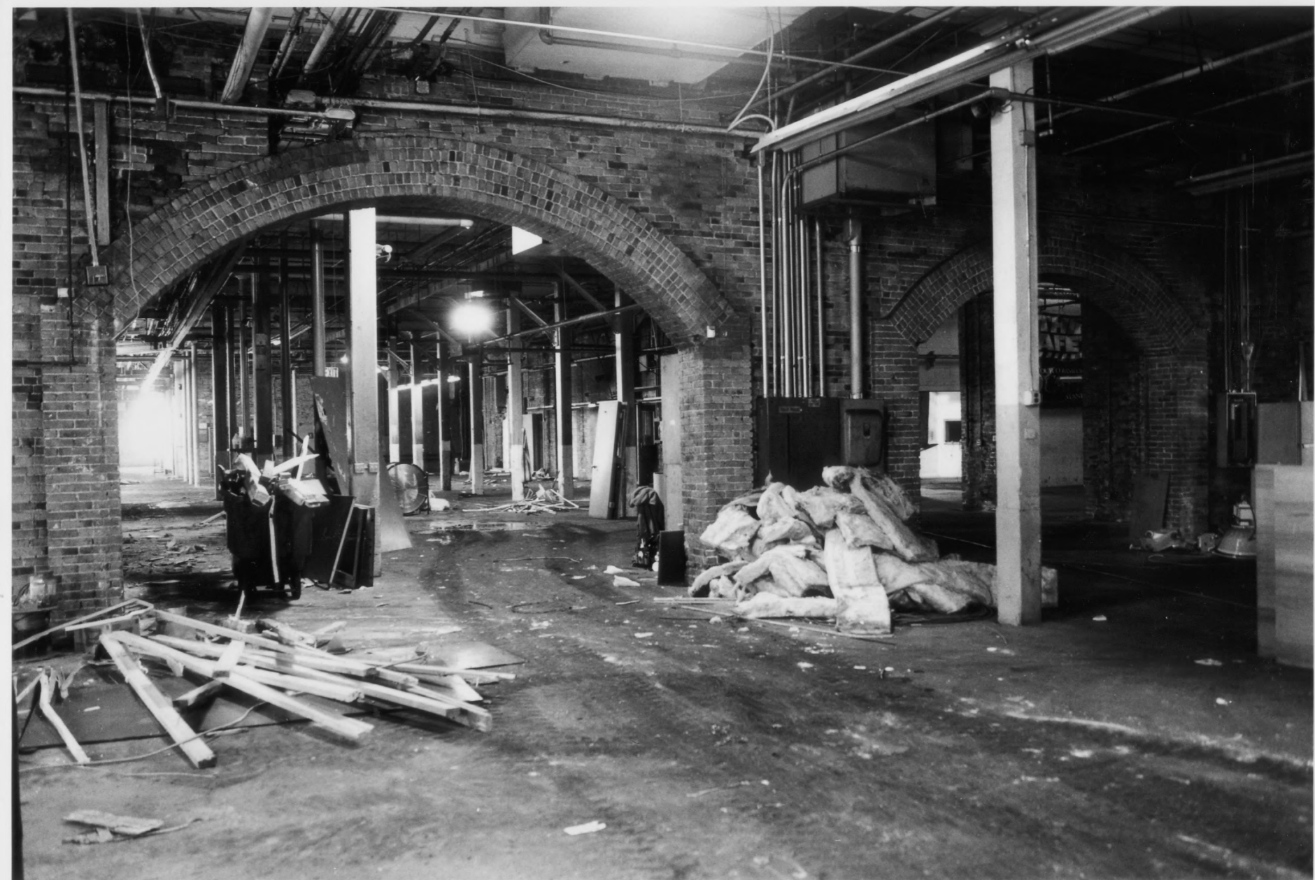
Interior Building 1A looking Southeast Rhode Island Tool Company Providence, Providence County, Rhode Island Photograph No. 15
