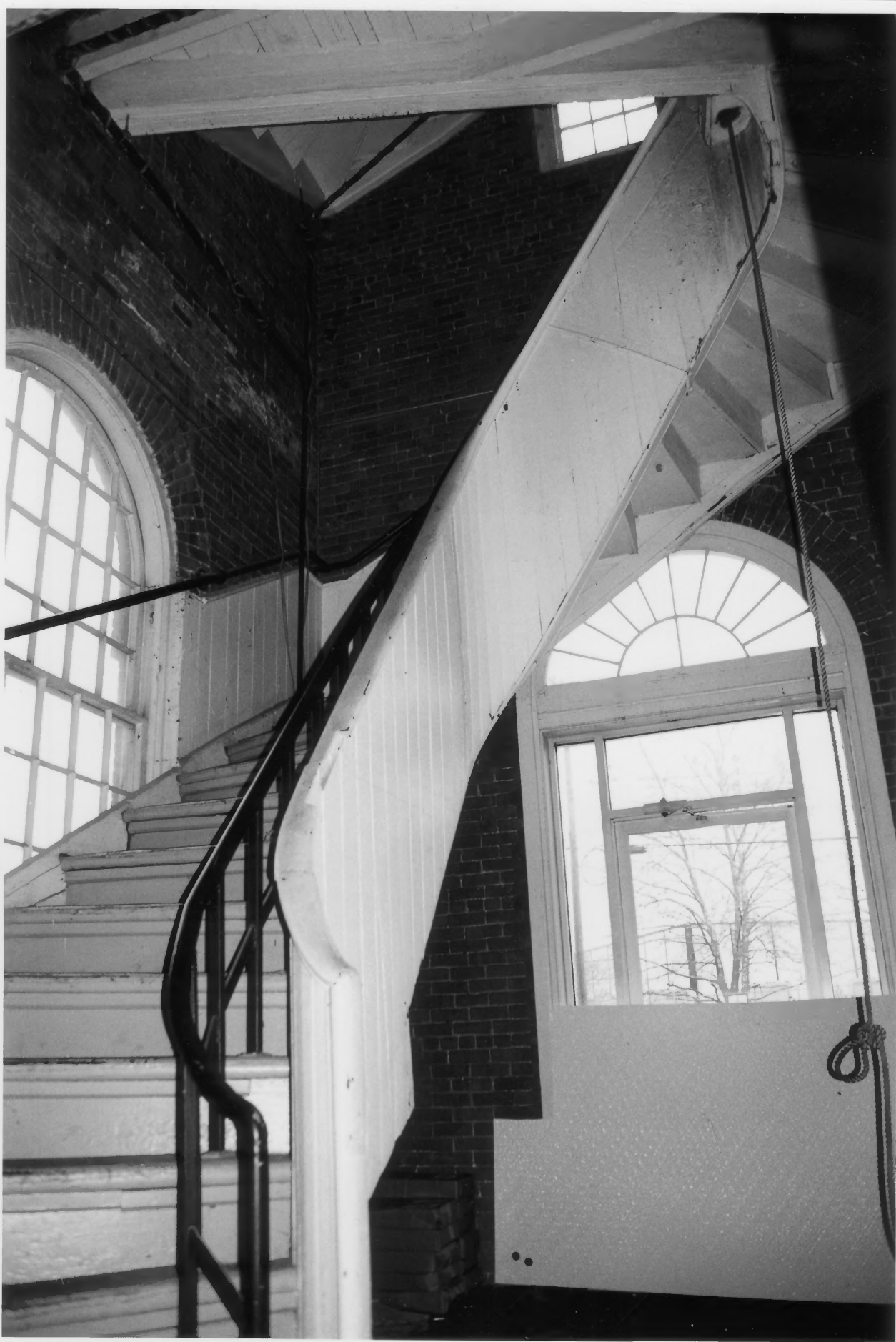
Interior First Floor of Building's Stair Tower Rhode Island Tool Company Providence, Providence County, Rhode Island Photograph No. 14
