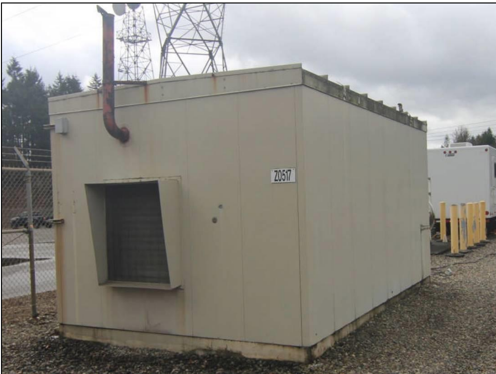
Photo 21 of 22: Engine Generator Building (1973), looking south. (WA_KingCounty_CovingtonSubstation_0021)
