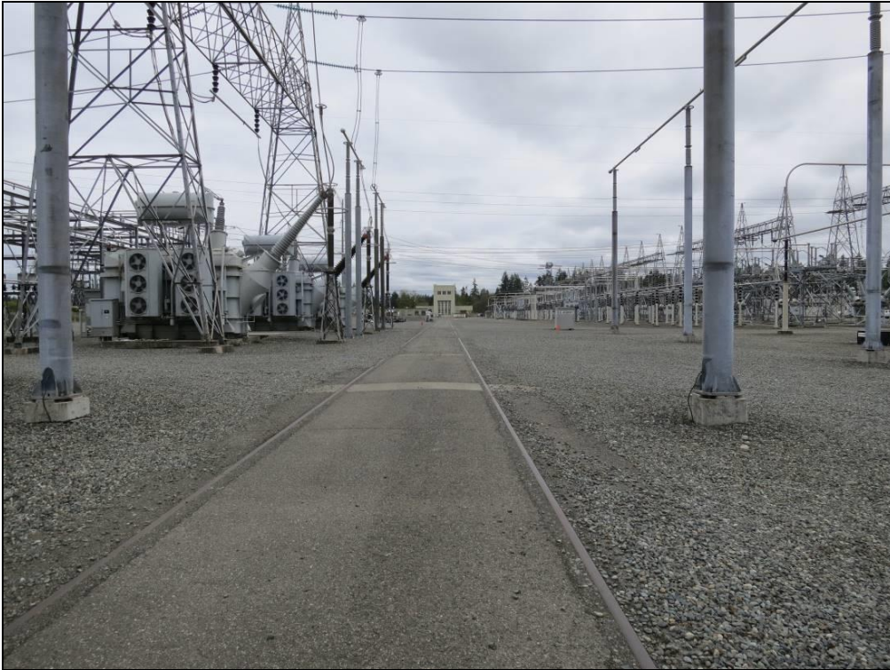
Photo 10 of 22: The Switchyard, Untanking Tower at center, looking northeast. (WA_KingCounty_CovingtonSubstation_0010)
