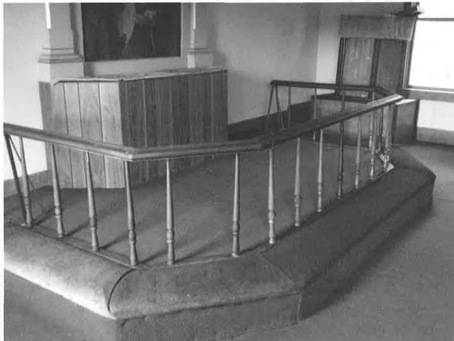
Detail of altar rail, platform and kneeling bench, View to the NNE towards the pulpit in background
