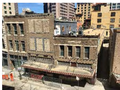
ID# 25b, 26, 26a, 27a, 27b Veramendi, Clegg, Kennedy, Little Savoy Buildings 118, 130, 134, 138 Soledad Contributing
