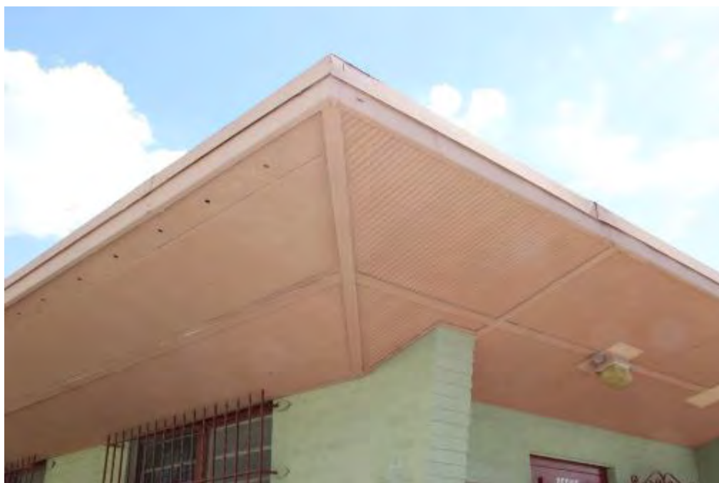
Photograph 18 – Enlarged view of reverse hip soffit at corner of Maintenance Building. Camera facing southwest. (June 28, 2016)
