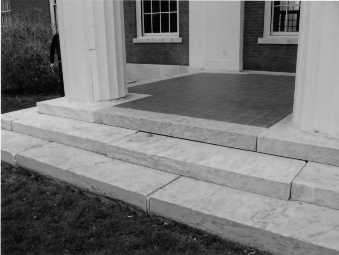
Photograph 0004: Eclectic Society House, Middletown, CT Marble stairs at the entrance portico on the west elevation; camera facing northeast
