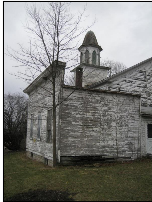
Figure 17. West elevation, showing 1891 session room in more detail. There is an outside entrance on the front elevation and what may have been a window at rear (January, 2017).
