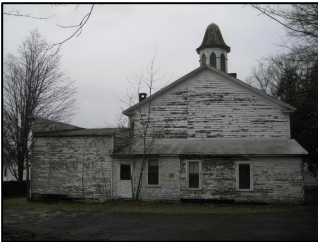
Figure 16. Rear (south) elevation with session room at left and kitchen at right (January, 2017).
