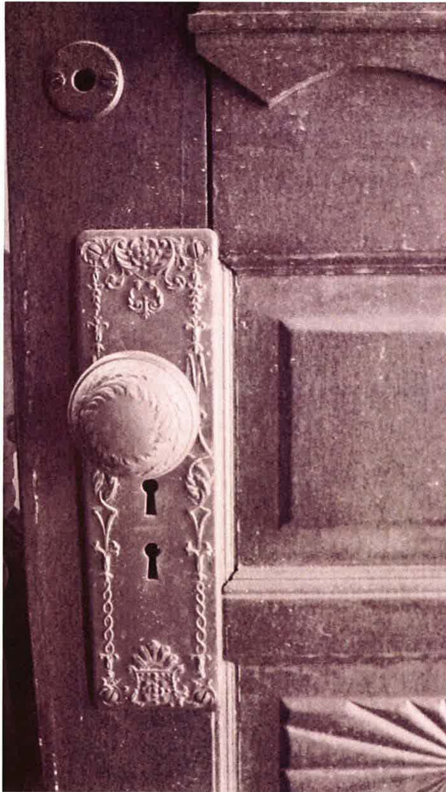
DE_Sussex County, Evans-Went House Original electroplated hardware, front door - main facade 08 of 14
