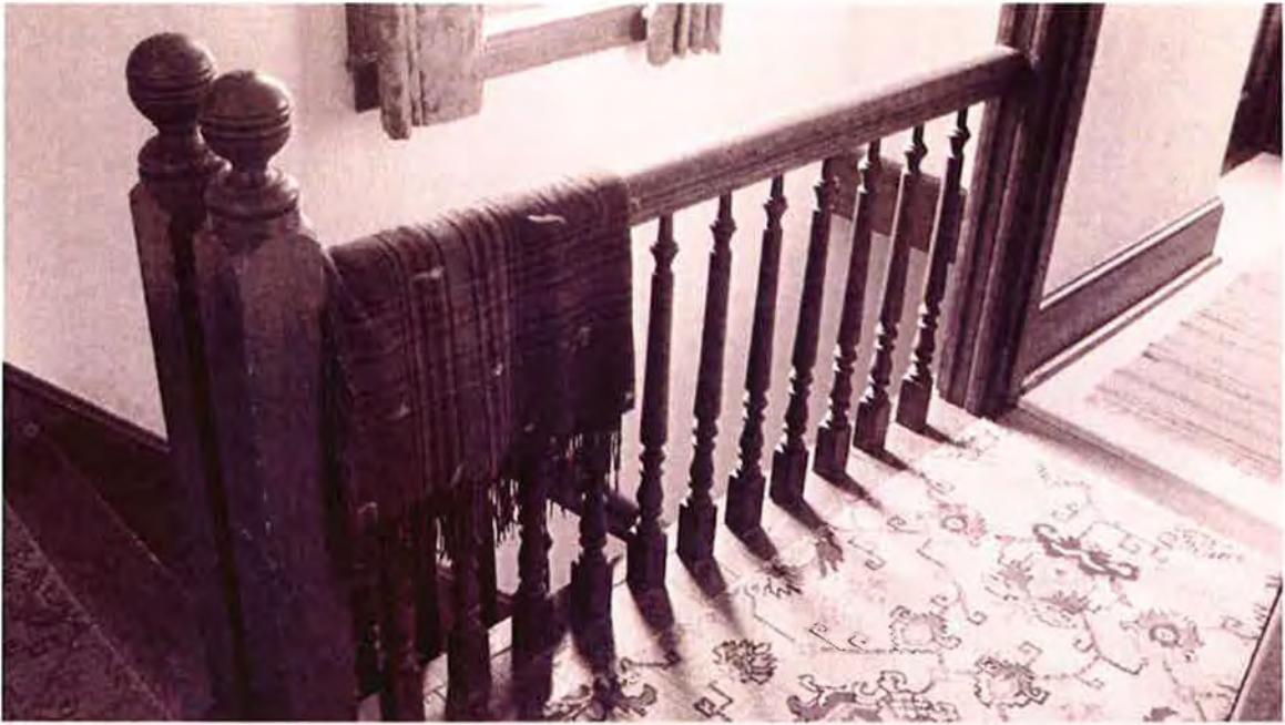
DE Sussex County Evans-West House Original second floor staircase with double newel posts, turned balusters, and molded handrail
