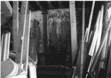
Figure 9 Current representative view of ground floor. The camera is positioned just inside the rear entrance (off camera at right) and facing south. The southwest corner of the building is behind the lumber at right. (Tallgrass Historians L.C., 2006)
