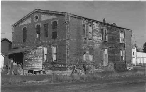
Figure 3 Current view of the west rear and the south side wall, looking northeast. (Tallgrass Historians L.C., 2006)
