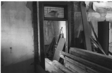
Figure 8 Current view of upper floor from stair landing, looking southeast through doorway into the southeast corner room. (Tallgrass Historians L.C., 2006)
