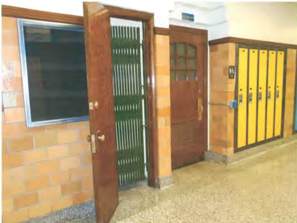
Figure 8 This interior ground floor view reflects a number of common features found in the 1934 building, including glazed tile lower walls trimmed by wood at the upper edge, terrazzo floors, arched-window wooden doors with divided lights, inset hallway lockers, and the ziggurat form over the inset door. Also visible here is a vault room with a security gate and, on the wall, a display case framed with white metal. Tallgrass Historians L.C., 2014
