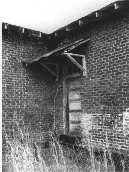
Entrance on the west façade of the east wing, view to northeast.
