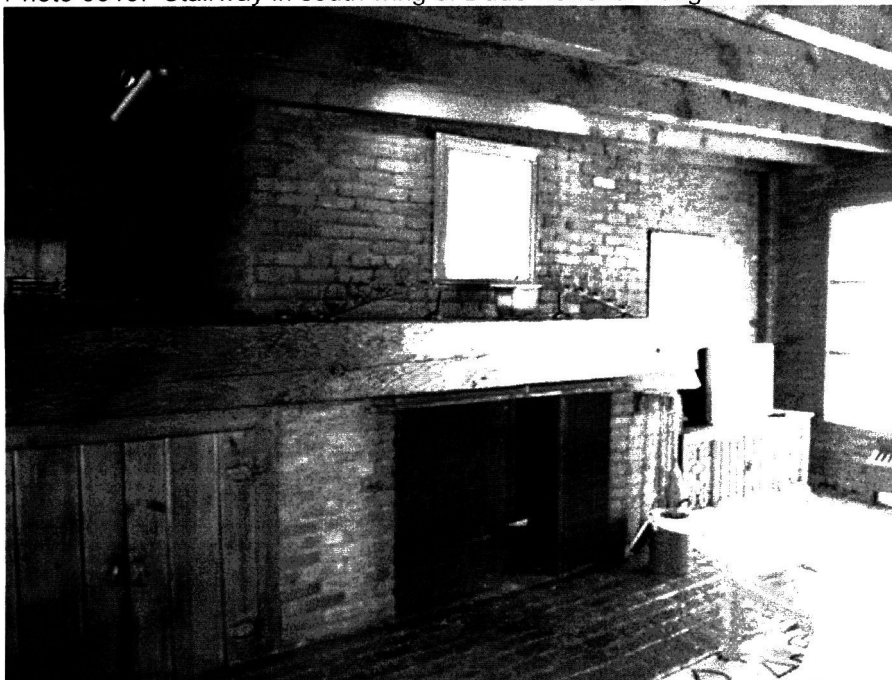
Photo 0020. Fire place in lounge area of Dude Rancher Lodge. View to the southeast.
