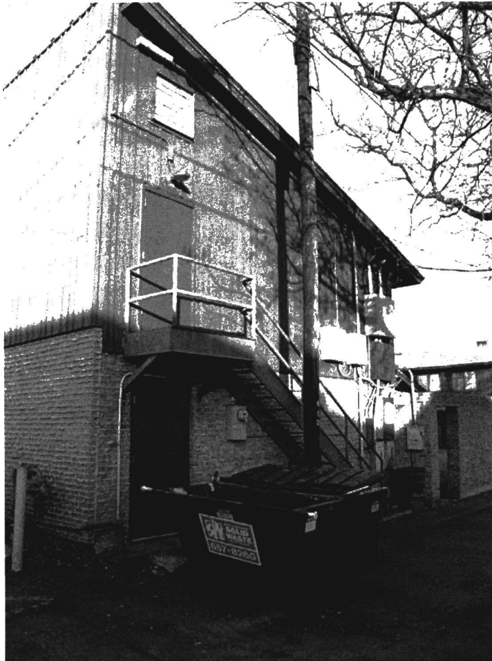
Photo 0006. Rear façade of south wing of Dude Rancher Lodge. View to the west.
