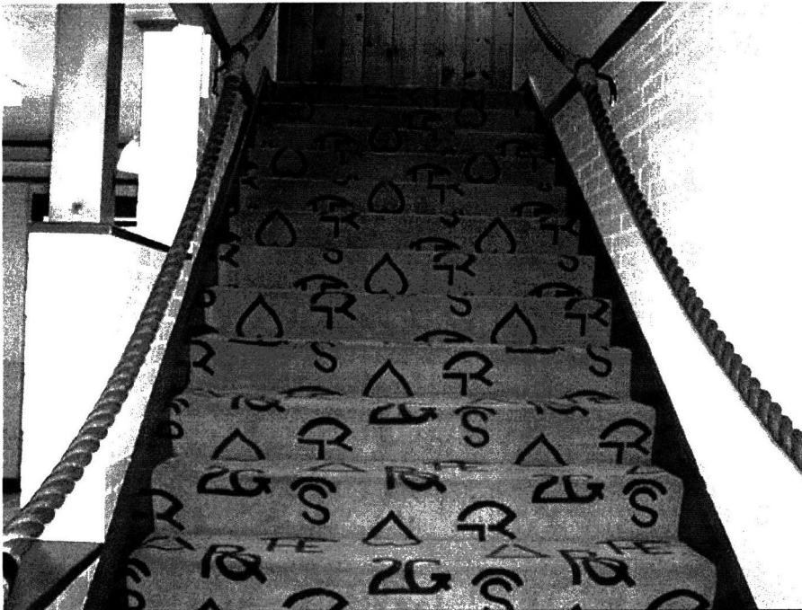
Photo 0019. Stairway in south wing of Dude Rancher Lodge. View to the south.
