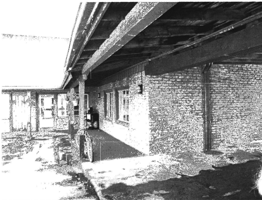
Photo 0015. Rear façade of Façade section of Dude Rancher Lodge. View to the south.
