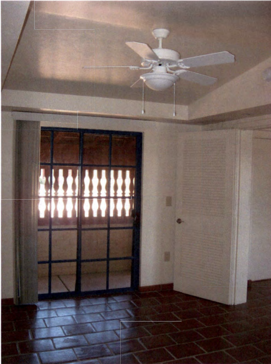
39. Original Building Group Typical bedroom addition that in-fills original carport yet retains original grilles and sense of space with a private patio. (Photo by Don W. Ryden of Ryden Architects, Inc., 2010)
