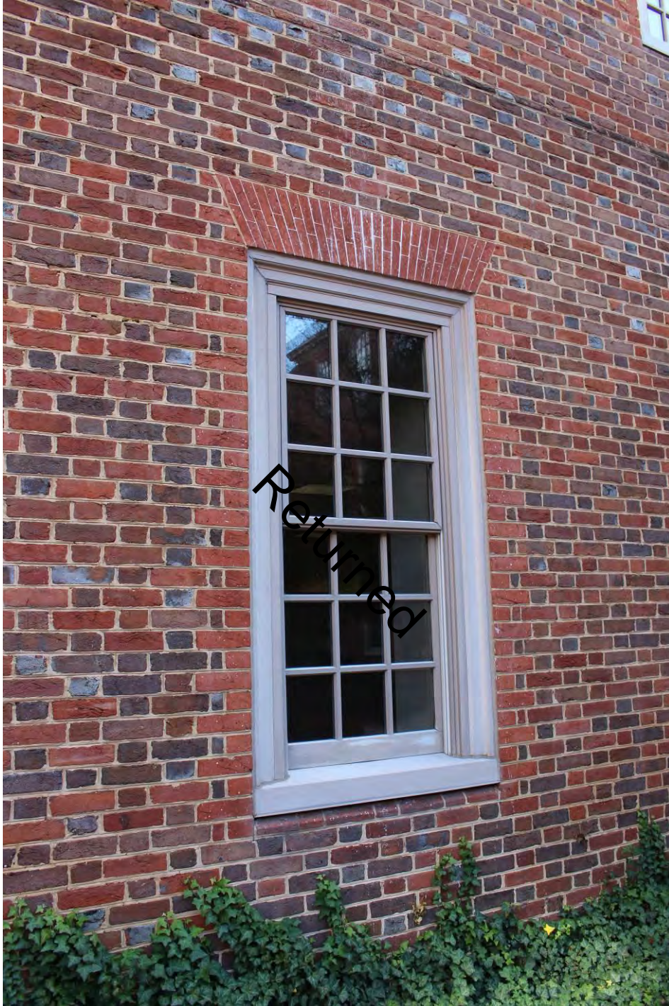
Photograph 18 of 22: Typical window of original 1950s section in south courtyard, facing southeast.
