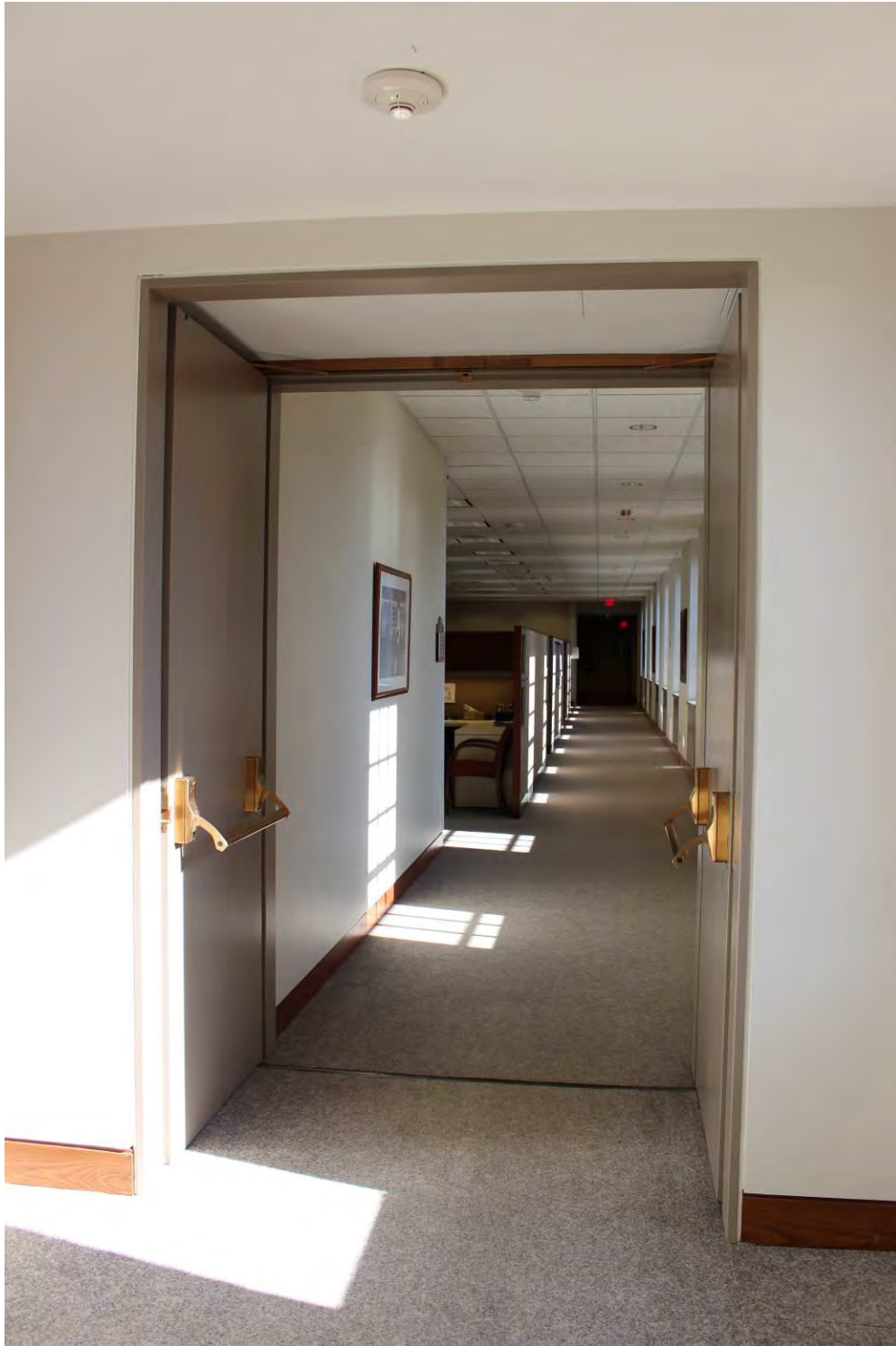
Photograph 22 of 26: Typical hallway and office space in north wing, second floor, facing east.
