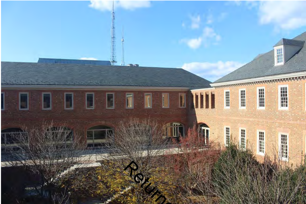
Photograph 15 of 22: View from second floor onto north courtyard showing connection between north wing and 1978 addition, facing west.
