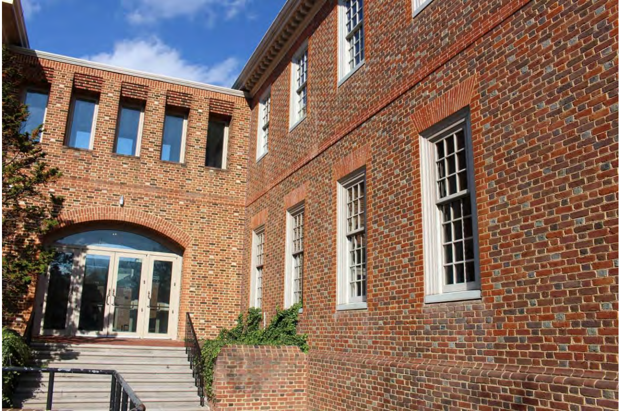
Photograph 9 of 26: West elevation of south wing and connection to 1978 addition, facing northeast. This connection and 1978 addition was demolished in 2019.
