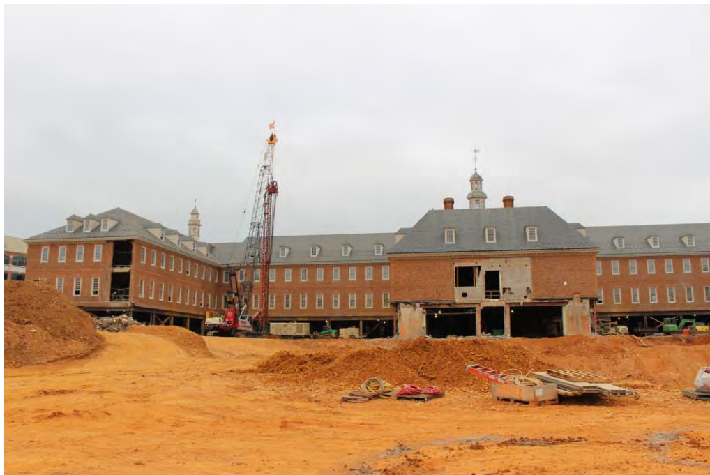
Photo 24 of 26: View looking east showing west elevation of center block and north end wing of building (2019)
