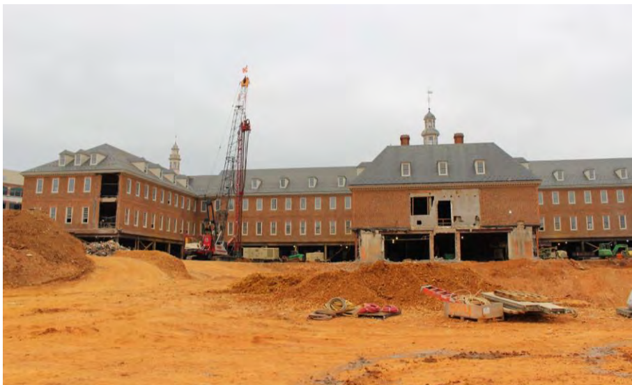
2019 view looking easterly showing west elevation of original building with 1978 addition removed
