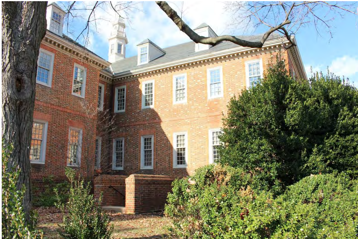
Photograph 10 of 26: South elevation of north wing with staircase to basement level, facing north.
