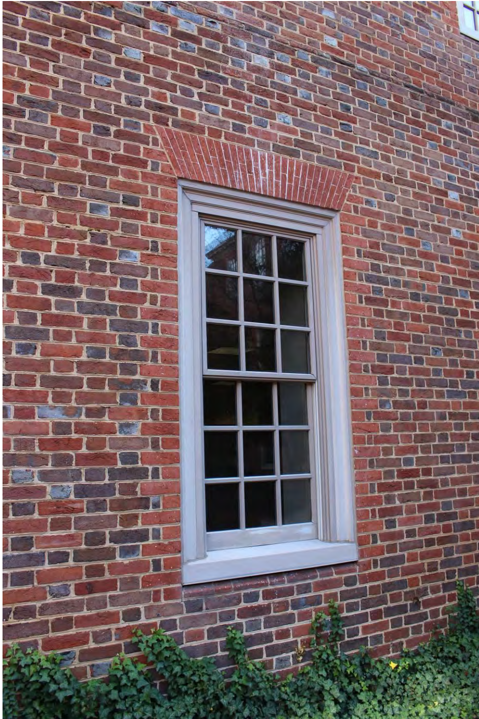
Photograph 18 of 26: Typical window of original 1950s section in south courtyard, facing southeast.
