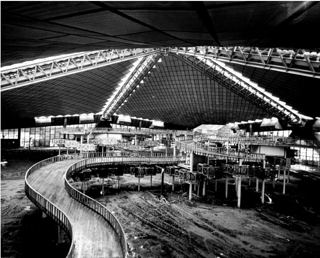
Interior of the Century 21 Coliseum, with roof still under construction, c. 1961 Museum of History & Industry, Seattle
