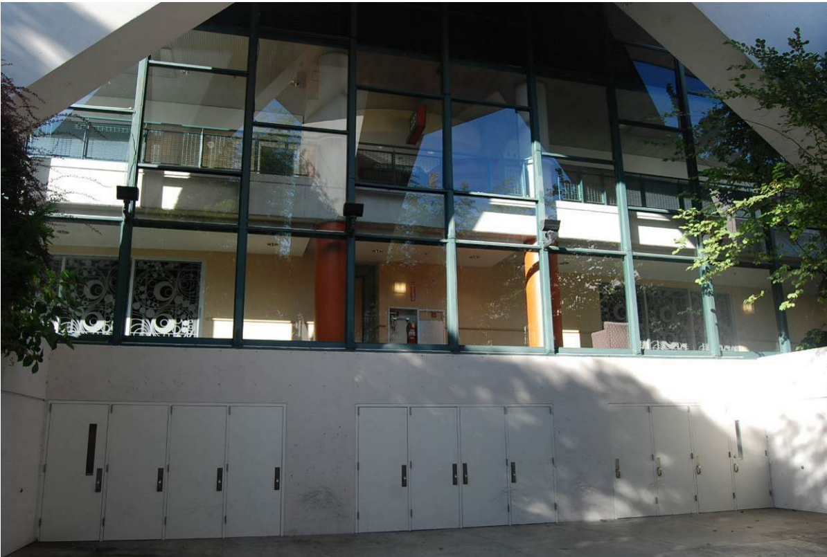
Photo 13 of 46 (WA_King County_Century 21 Coliseum_0013) – October 2017 Detail view of the curtain wall and exit doors on the south façade, facing north
