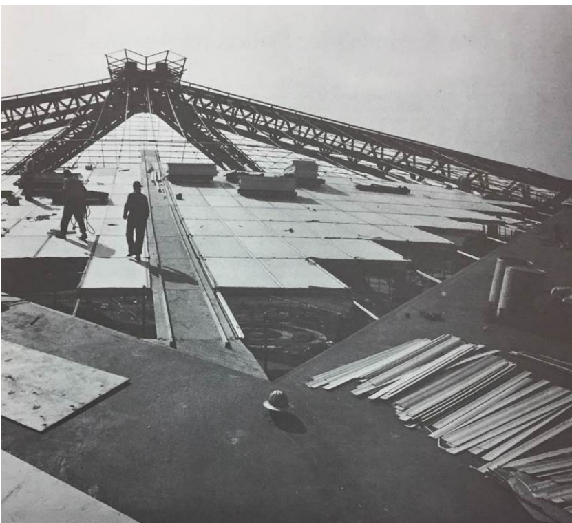
Century 21 Coliseum, installation of roof panels, 1962 Materials and Methods: Century 21's Coliseum Roof, pg. 181, March 1962
