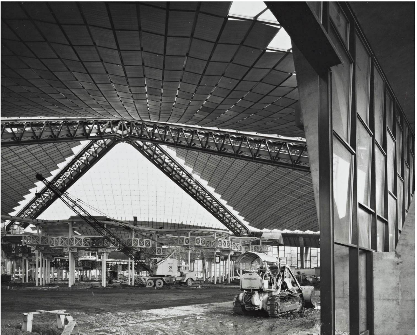
Century 21 Coliseum under construction showing portion of exterior curtain wall. Department of Archaeology & Historic Preservation
