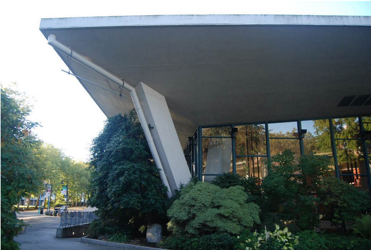
Photo 22 of 46 (WA_King County_Century 21 Coliseum_0022) – October 2017 Detail view of the entrance on the east façade and V-shaped concrete pier, facing south
