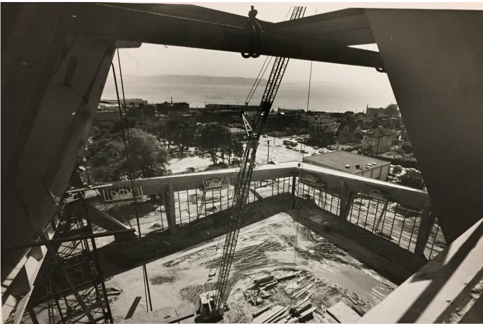
Century 21 Coliseum under construction, January 9, 1961 Municipal Reference Library, Branch of Seattle Public Library
