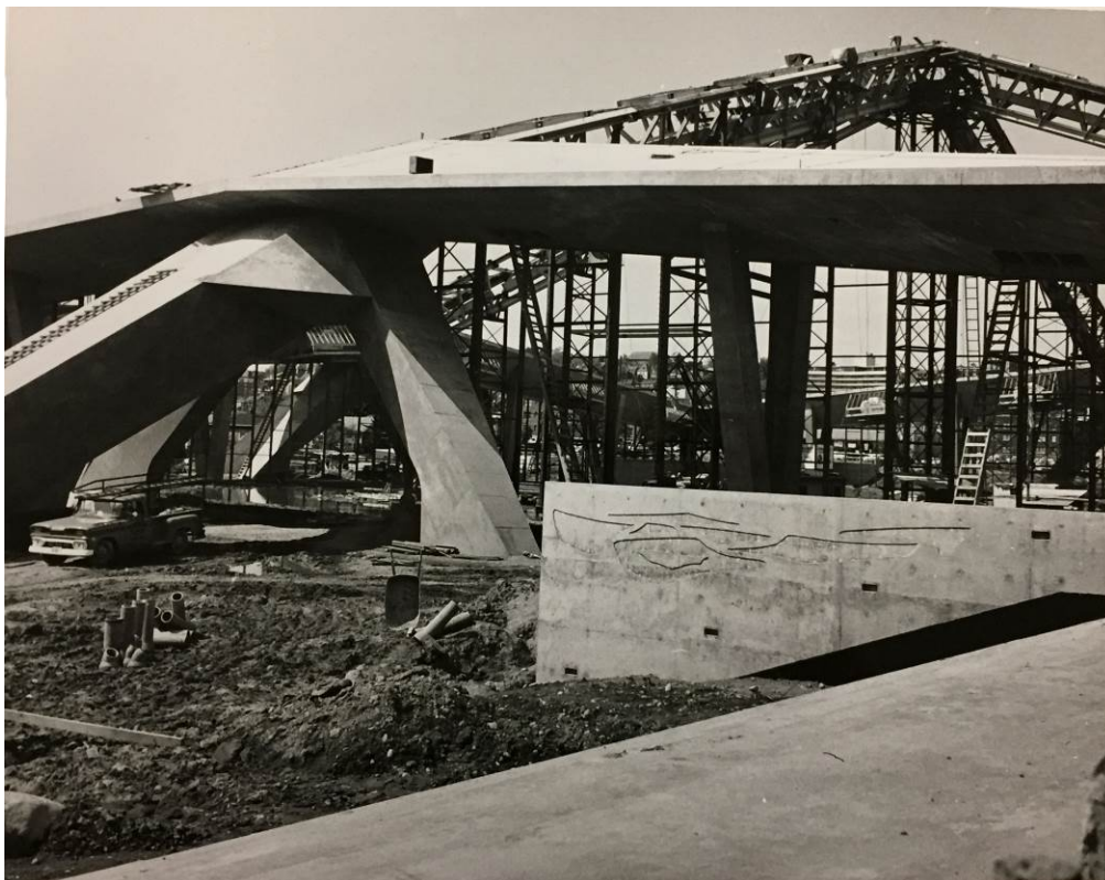
Century 21 Coliseum under construction, January 9, 1961 Municipal Reference Library, Branch of Seattle Public Library
