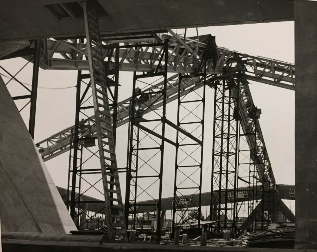
Century 21 Coliseum under construction, January 9, 1961 Municipal Reference Library, Branch of Seattle Public Library
