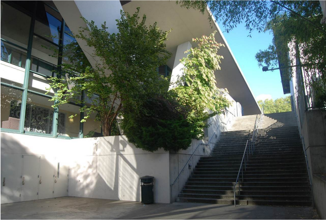
Photo 10 of 46 (WA_King County_Century 21 Coliseum_0010) – October 2017 Overall view of the south façade and stairs, facing northeast
