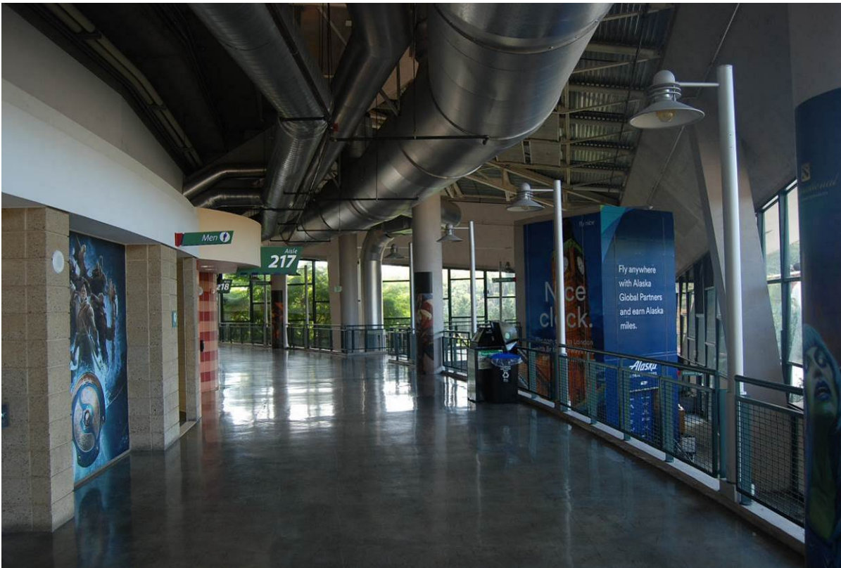
Photo 39 of 46 (WA_King County_Century 21 Coliseum_0039) – October 2017 View of the west side of the upper concourse level, facing south
