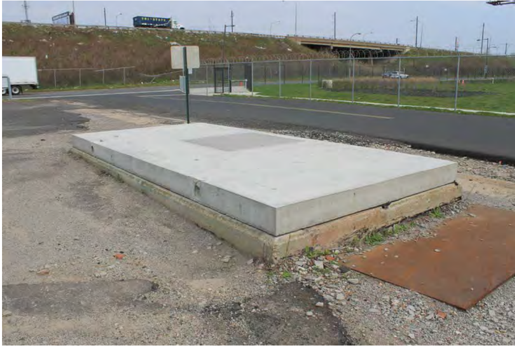
Photograph 1: View of one of the historic openings to the underground utilities network, facing northeast. Building No. 72 (tunnel entrance) historically covered this opening. Building No. 72 was demolished c.2007.
