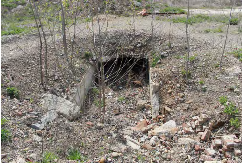
Photograph 3: View of tunnel opening likely leading into the underground utilities network, facing southeast.
