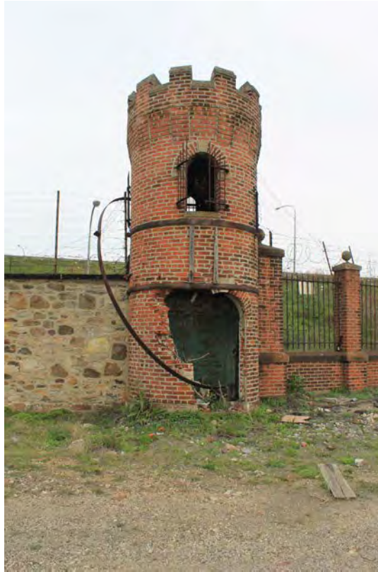
Photograph 11: View of the Machine Gun Tower (Building No. 49), facing northeast. Note the missing brick to the top left side of the doorway.
