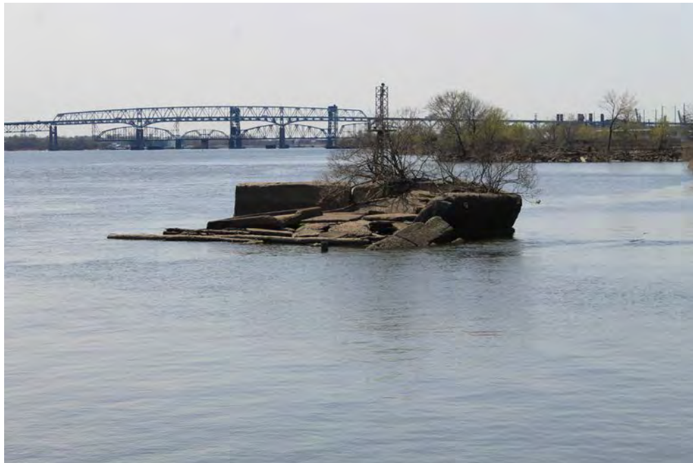
Photograph 14: View of the Building 409 (Laboratory Storage) ruins within the Delaware River, facing southwest. Note the piled collapsed sections and the tree growing through the concrete.
