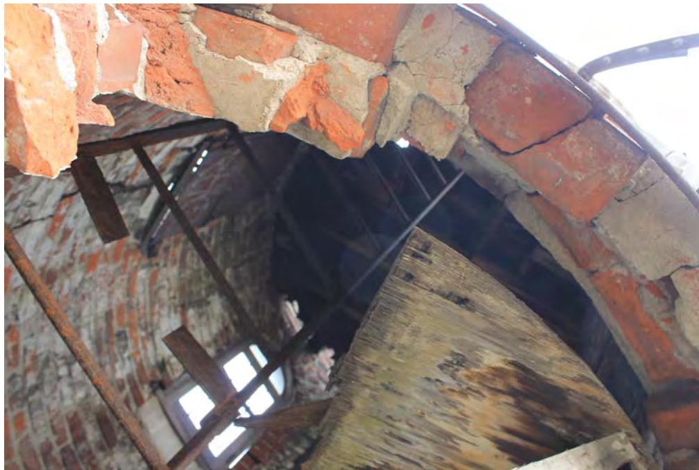
Photograph 12: View of the interior of the Machine Gun Tower (Building No. 49). Note the collapsed state of the wood floor (front right) and the holes in the upper floor just to the left of center.
