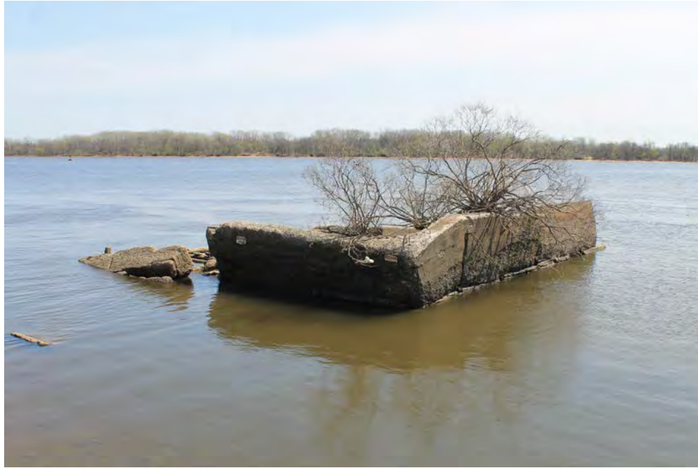
Photograph 13: View of the Building 409 (Laboratory Storage) ruins within the Delaware River, facing southeast. Note the collapsing wall to the left.
