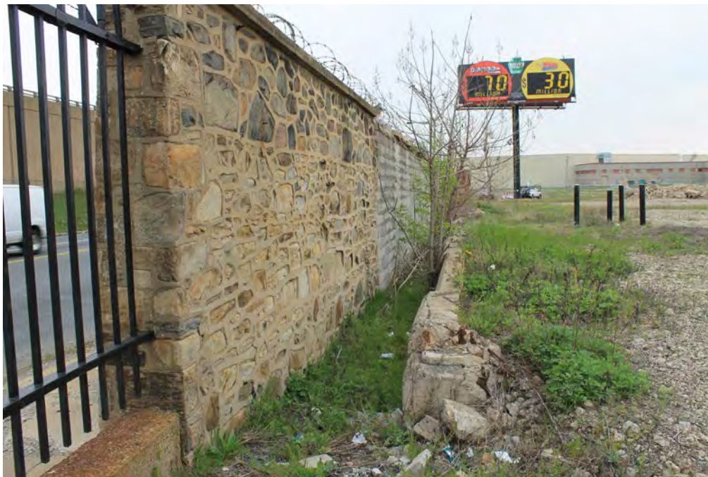
Photograph 4: View of the foundation remnants of Building No. 44 (General Purpose Administration Building), facing east. Note the concrete block infill within the Tacony Street boundary wall near the center of the photo. Building No. 44 was demolished c.2010.
