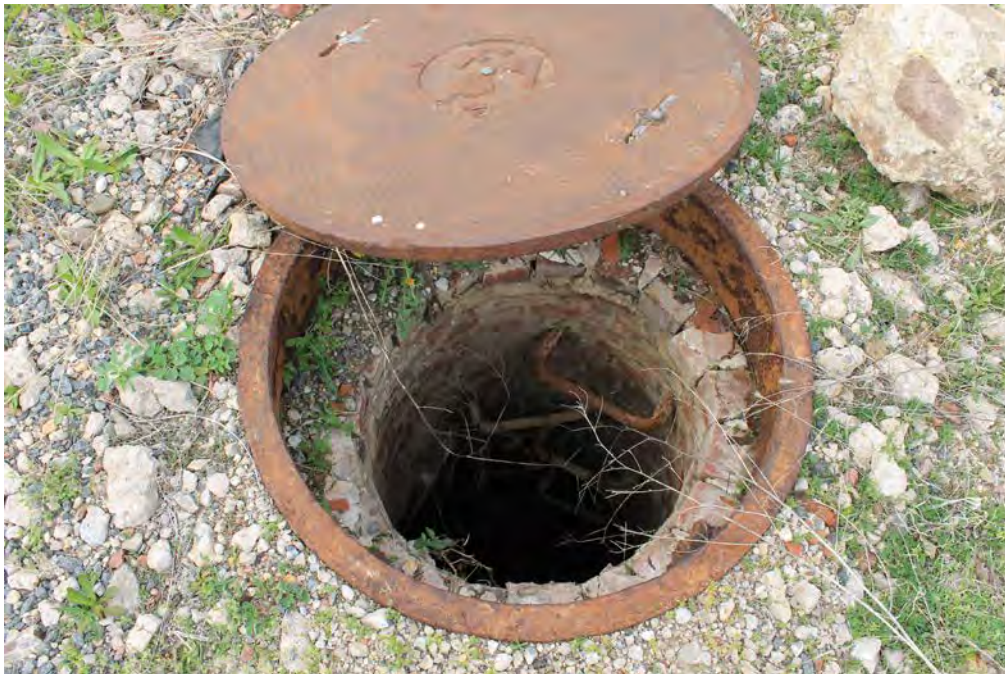
Photograph 2: View of a manhole leading to the underground utilities network and cover, facing southwest. Note the brick lining of the manhole and the "F A P" on the cover.
