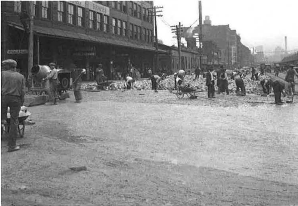
Figure 33: 9 April 1929 – Looking southwest along Pike Street (Smallman) toward downtown from 21st Street, showing men paving street. Image shows 2000 Smallman Street at left.
