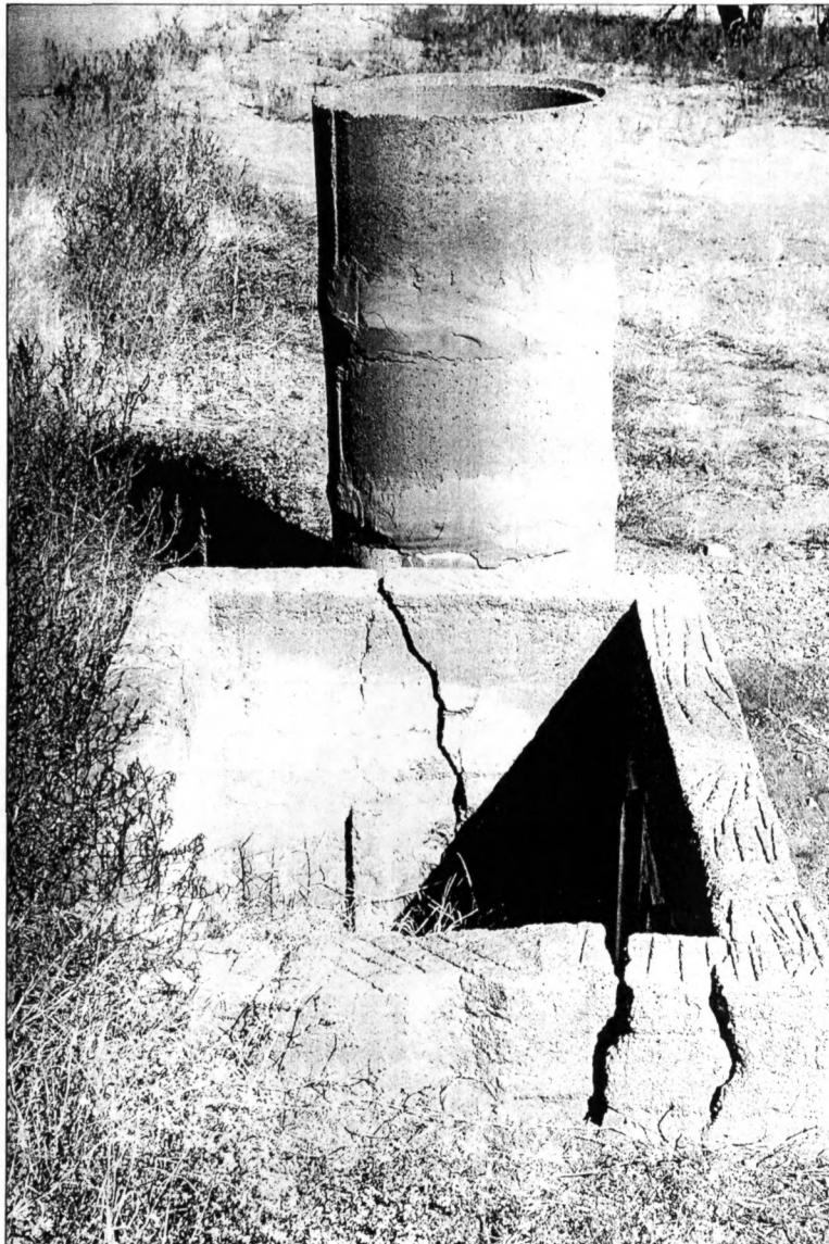
Figure 36. Concrete gate boxes (one rectangular, one cylindrical) for buried concrete irrigation pipeline, located on west side of ranch property midway between the Canal Head and South Residential Clusters.
