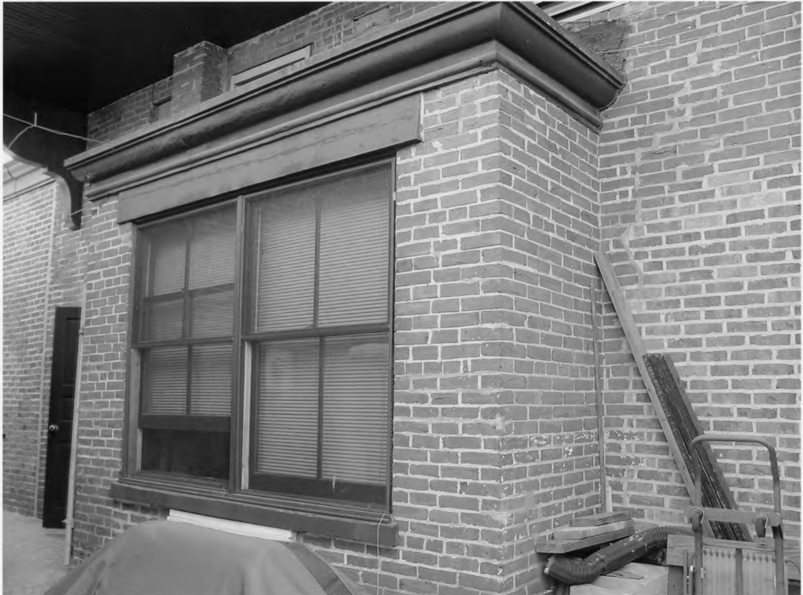
Water Witch Steam Fire Engine Company No.5 - Wilmington southwest elevation looking north New Castle County, DE
