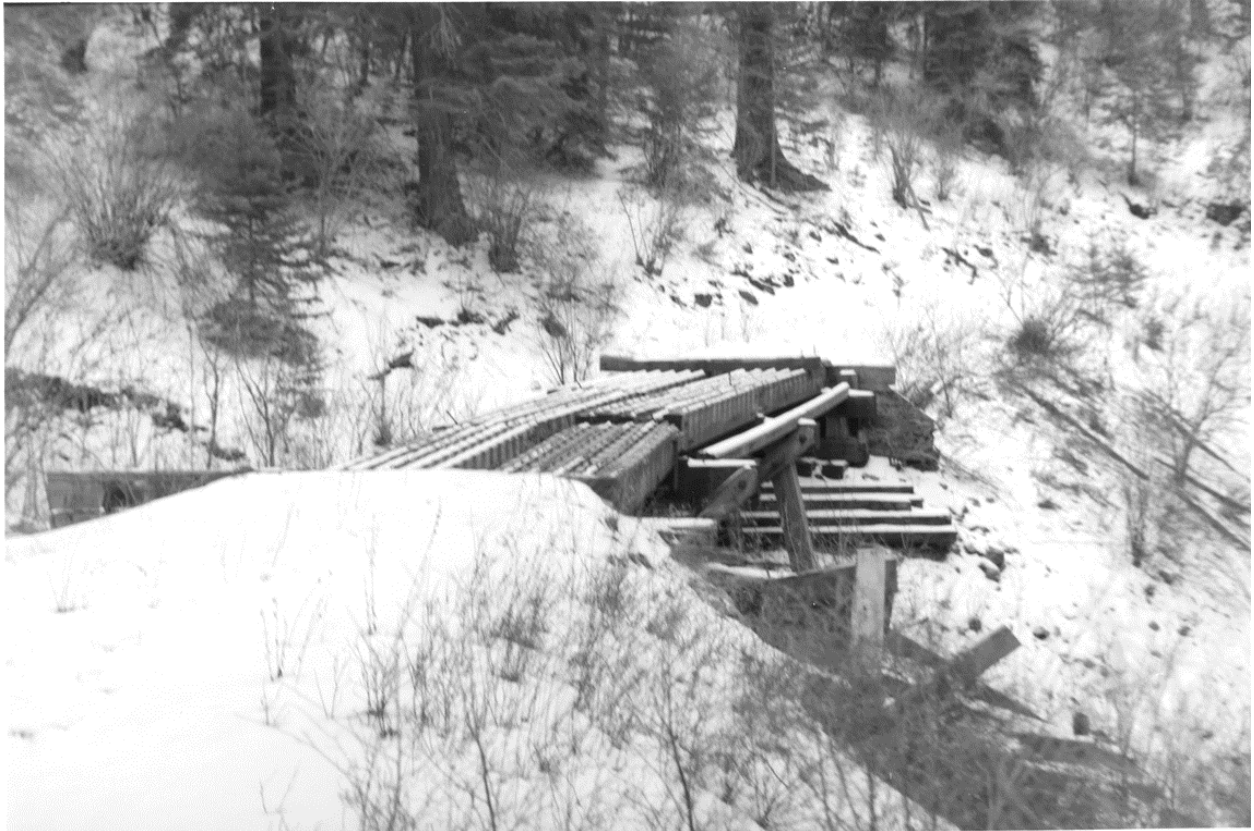
Figure 4. Bridge A 249 in 1959, with exposed stringers.
