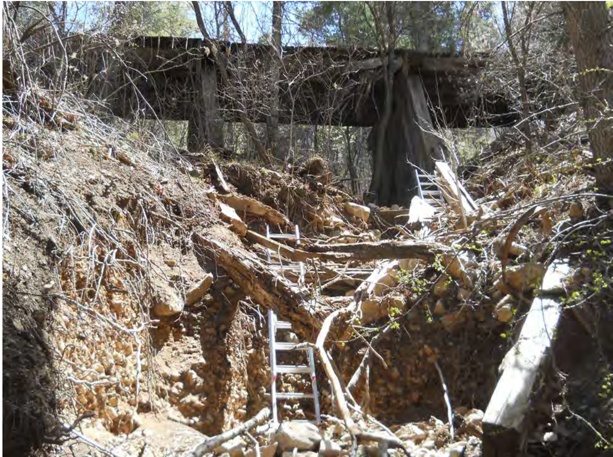
17 of 17. Bridge A 249, with remains of water control structure in foreground, photographer facing south.
