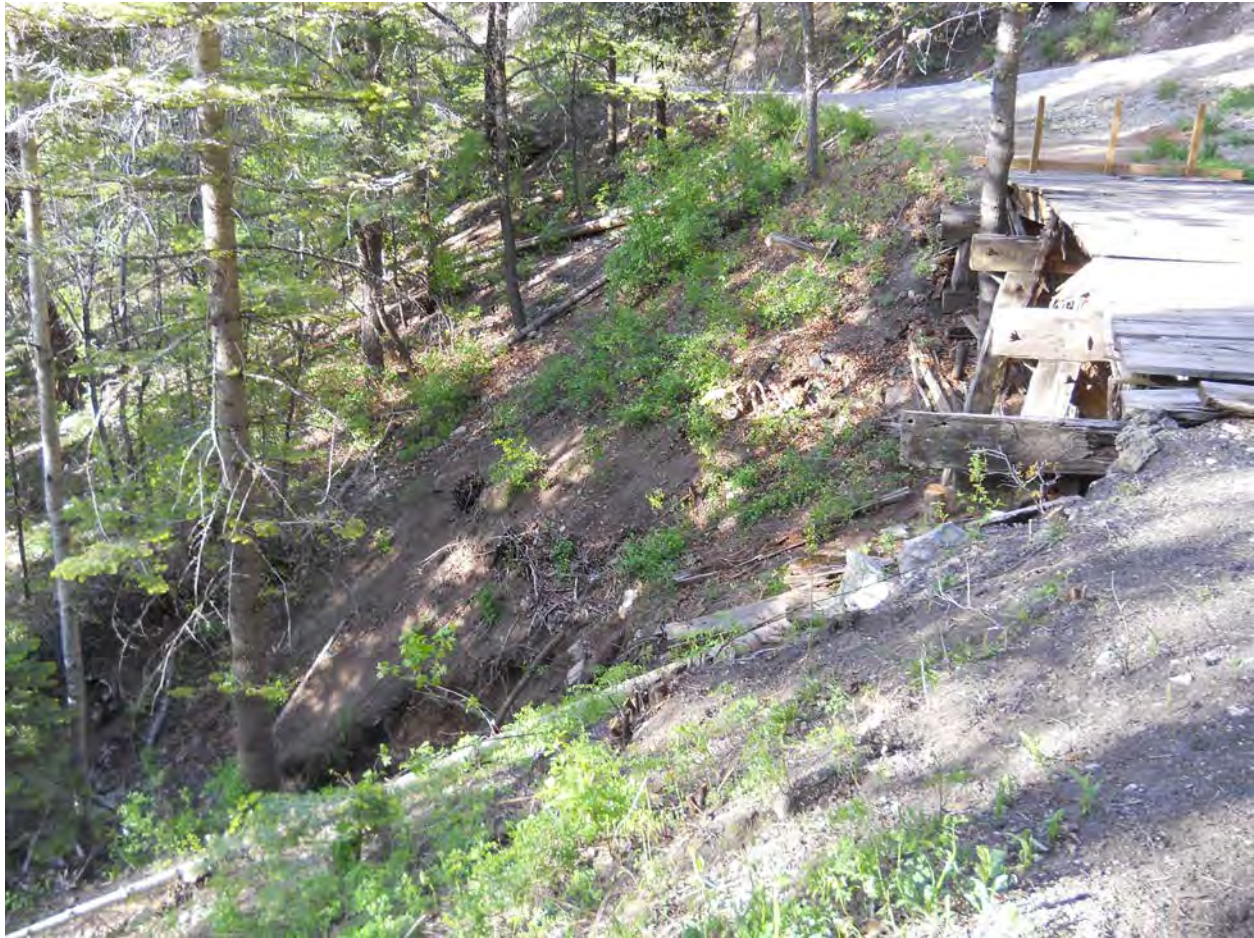
5 of 17. Bridge A 249 and down slope with remains of water control structure, photographer facing northeast.
