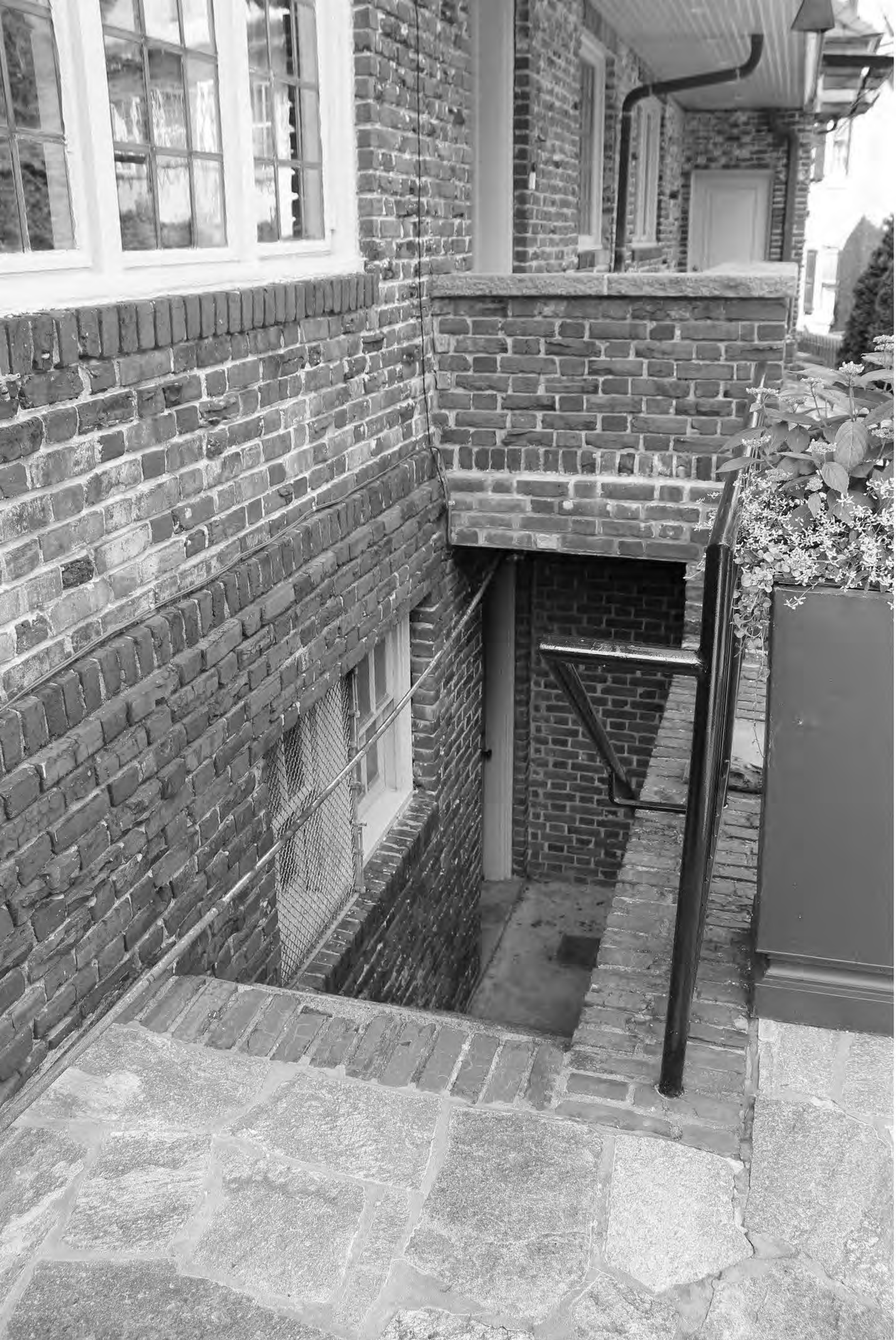
Jackson-Wilson House _ New Castle County _ DE Detail of stair to basement entrance, facing east
