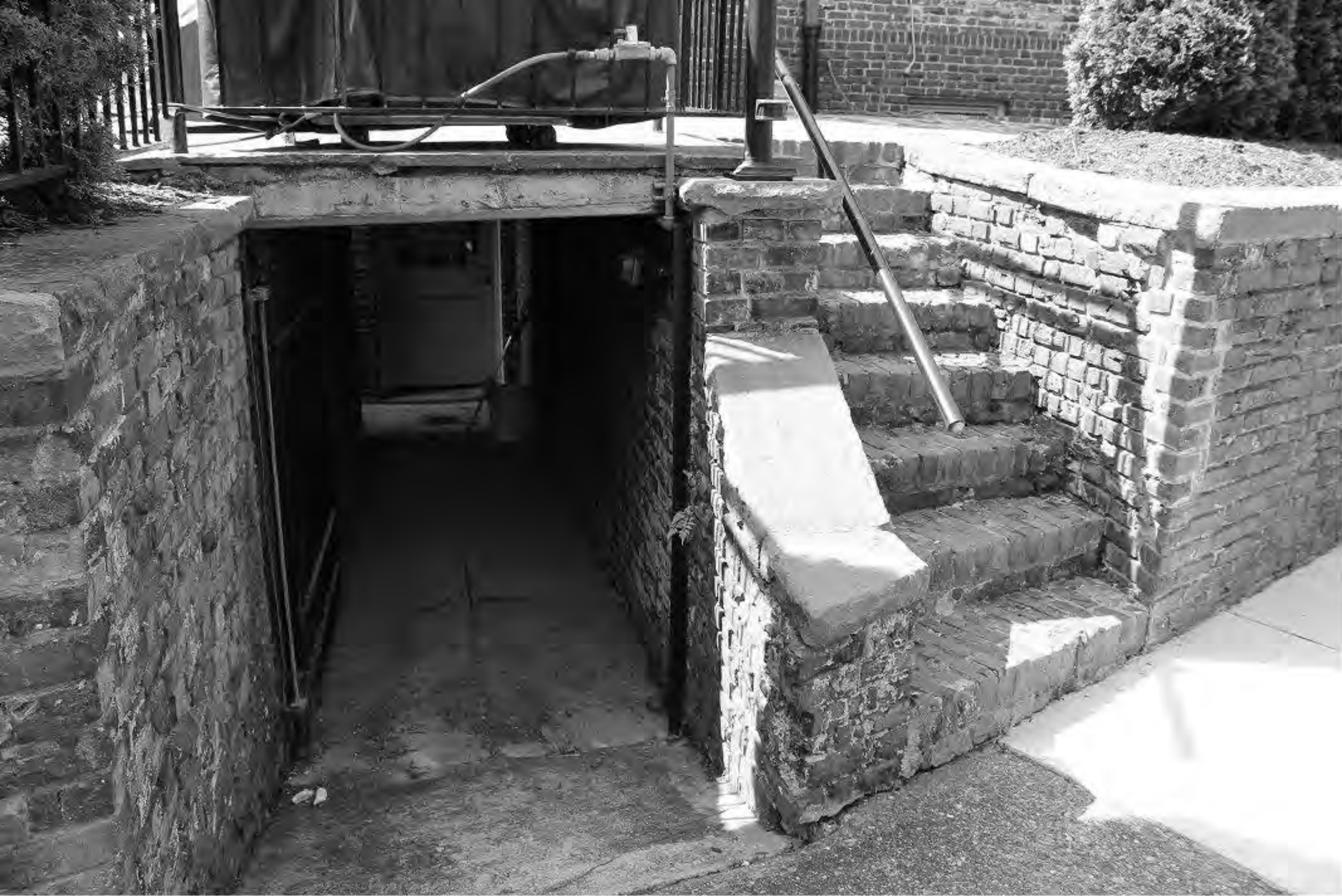
Jackson-Wilson House _ New Castle County _ DE Below grade tunnel entrance to basement and stairs to rear patio, facing northeast
