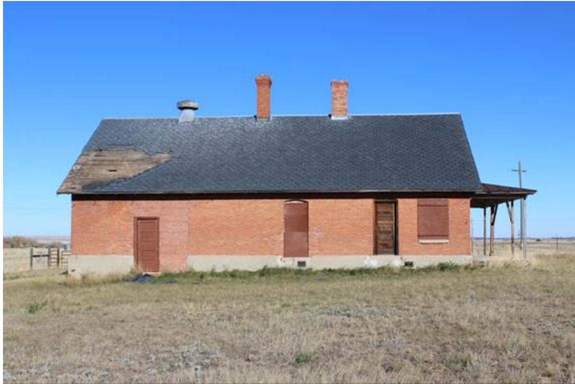
DBL. CALVARY STABLE GUARD/SHOP BLDG. (BLDG. #92, EAST GRANARY), WEST ELEVATION, VIEW TO THE NORTHEAST MT_HillCounty_FortAssinniboine_0021
